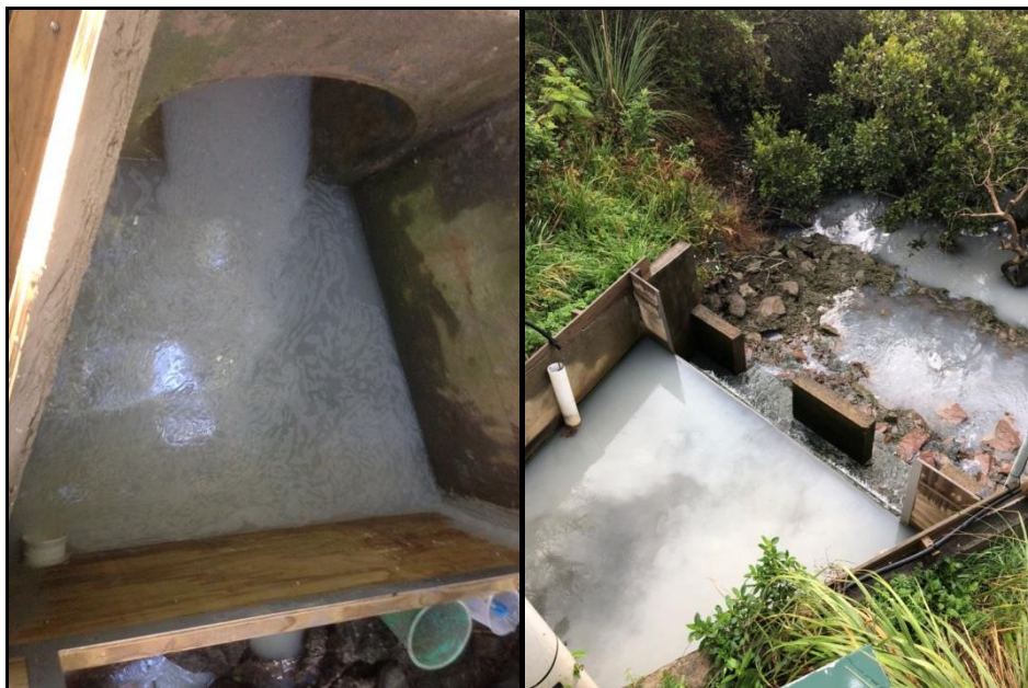
Figure 5. Two discharge events observed when monitoring staff were onsite during dry weather. Left is Akatea Road and right is Timothy Place
