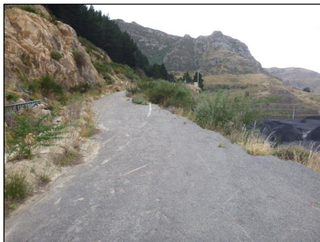
Figure 6: Damage to the road near Windy Point due to a slip removing a retaining wall below the road
