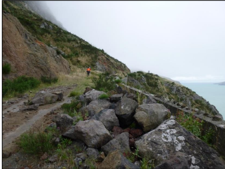
Figure 1: View of rockfall damage to Sumner Road (early 2016)
