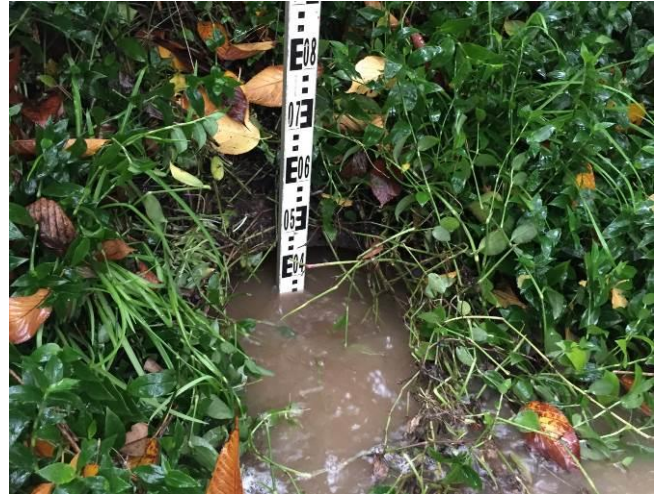
Figure 2-4 Insufficient hydraulic capacity for design flows demonstrated by submerged inlet during typical rainfall event
