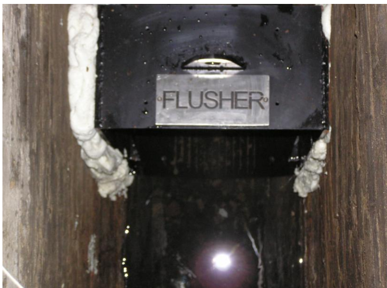
Figure 5 – A Flusher installed into a 525mm diameter wastewater sewer manhole.
