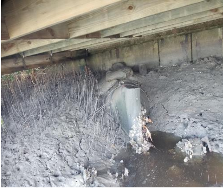
Older style duckbill valve damaged and non-functioning due to oyster growth and general material degradation.
