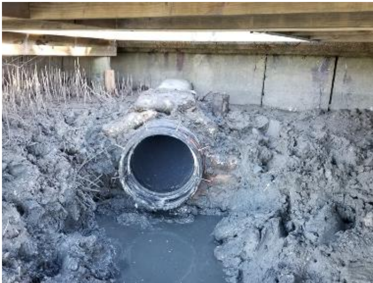
WaStop valve installed inside the existing pipe after removal of the duckbill.
