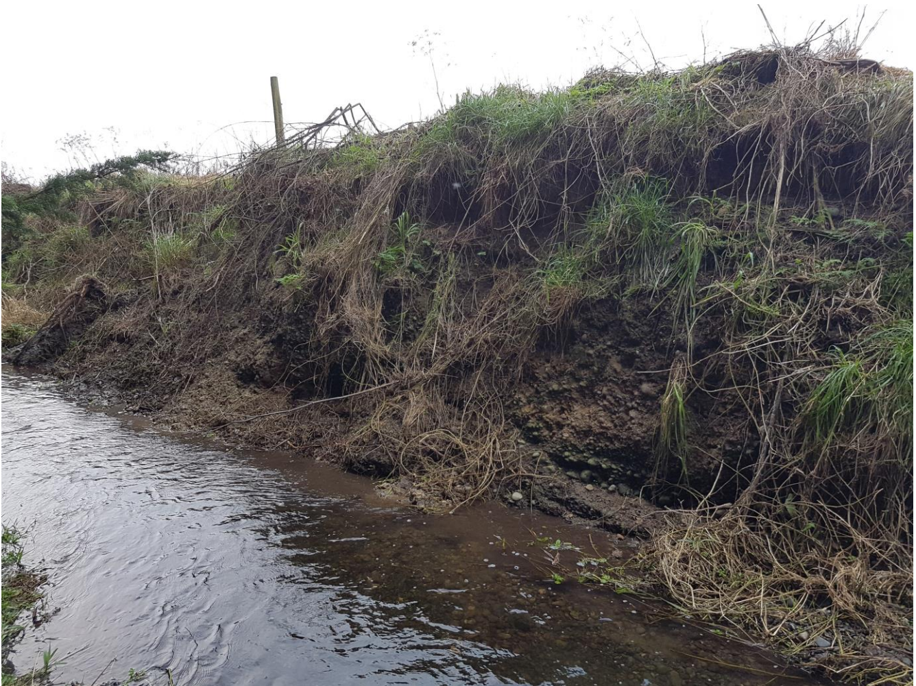
Photograph 1: View of Snake Creek Bank Erosion Prior to the Works
