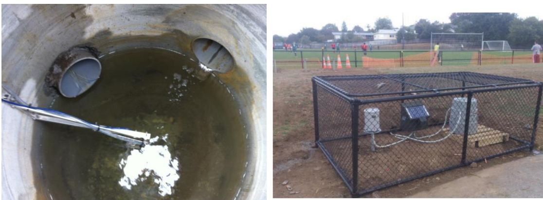
Plate 1 (left): View inside the manhole where monitoring equipment was located. Exit pipe orifice is top left, one sub-surface drain can be seen entering at top right.
