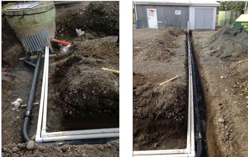
Photograph 11: New rising main to new treatment equipment installed within existing building
