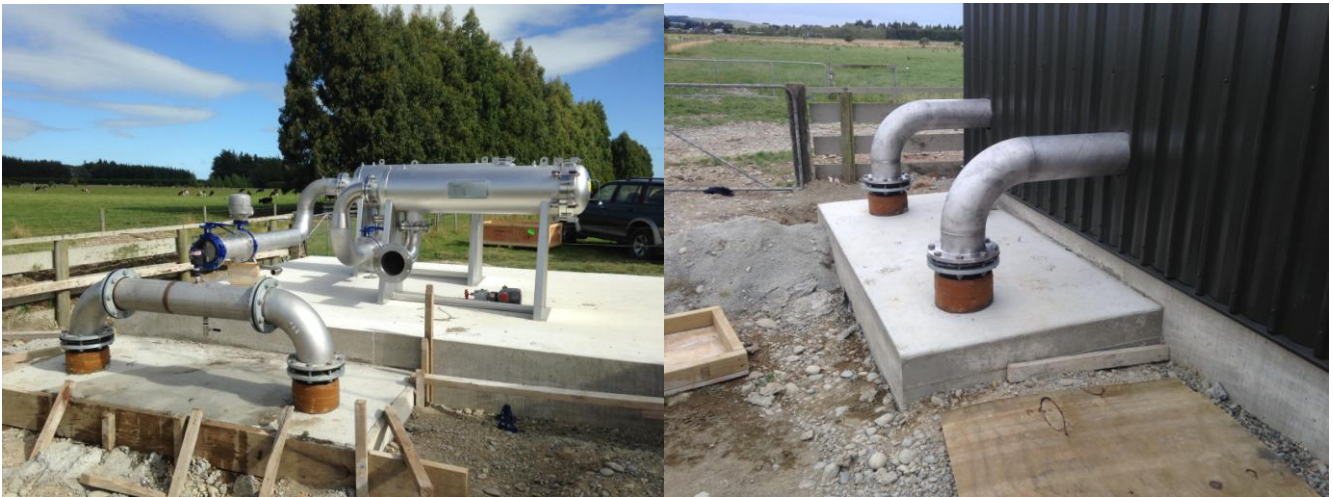
Photograph 10: Left hand photo shows temporary arrangement of rising main during construction of filter building. Right hand photo shows the final configuration
