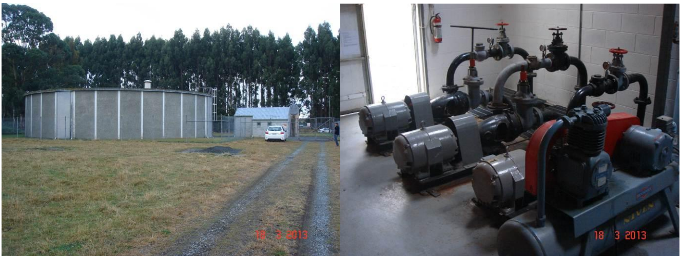
Photograph 4: Winton Water Treatment Plant and Secondary Pumps (Existing)
