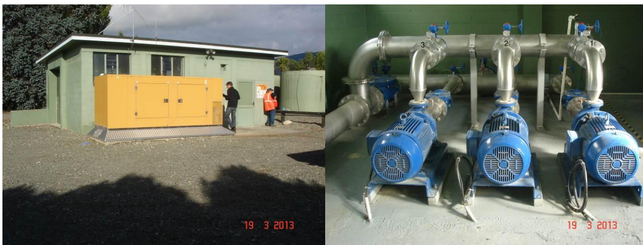
Photograph 1: Te Anau Water Treatment Plant and Secondary Pumps (Existing)
