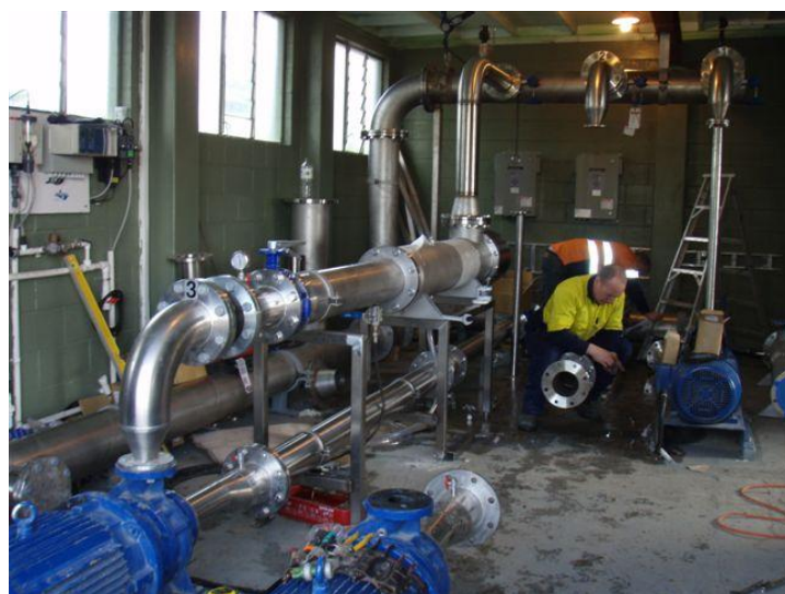
Photograph 9: Update in progress – first pump in new configuration, second pump being worked on and third pump with temporary connection to relocated discharge manifold
