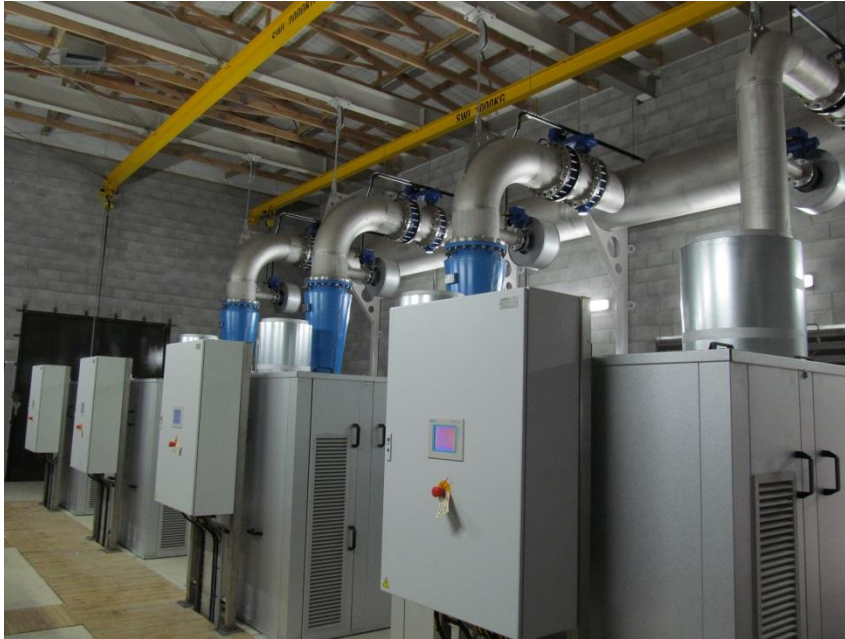
Photograph 2: Newly installed Siemens blowers
