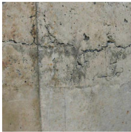
Figure 3: Typical Cement Cold Joint
