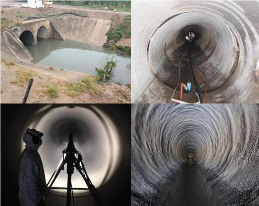
Figure 9: Images from the jobsite for the Rado Storm Drain; McAllen, TX. USA
