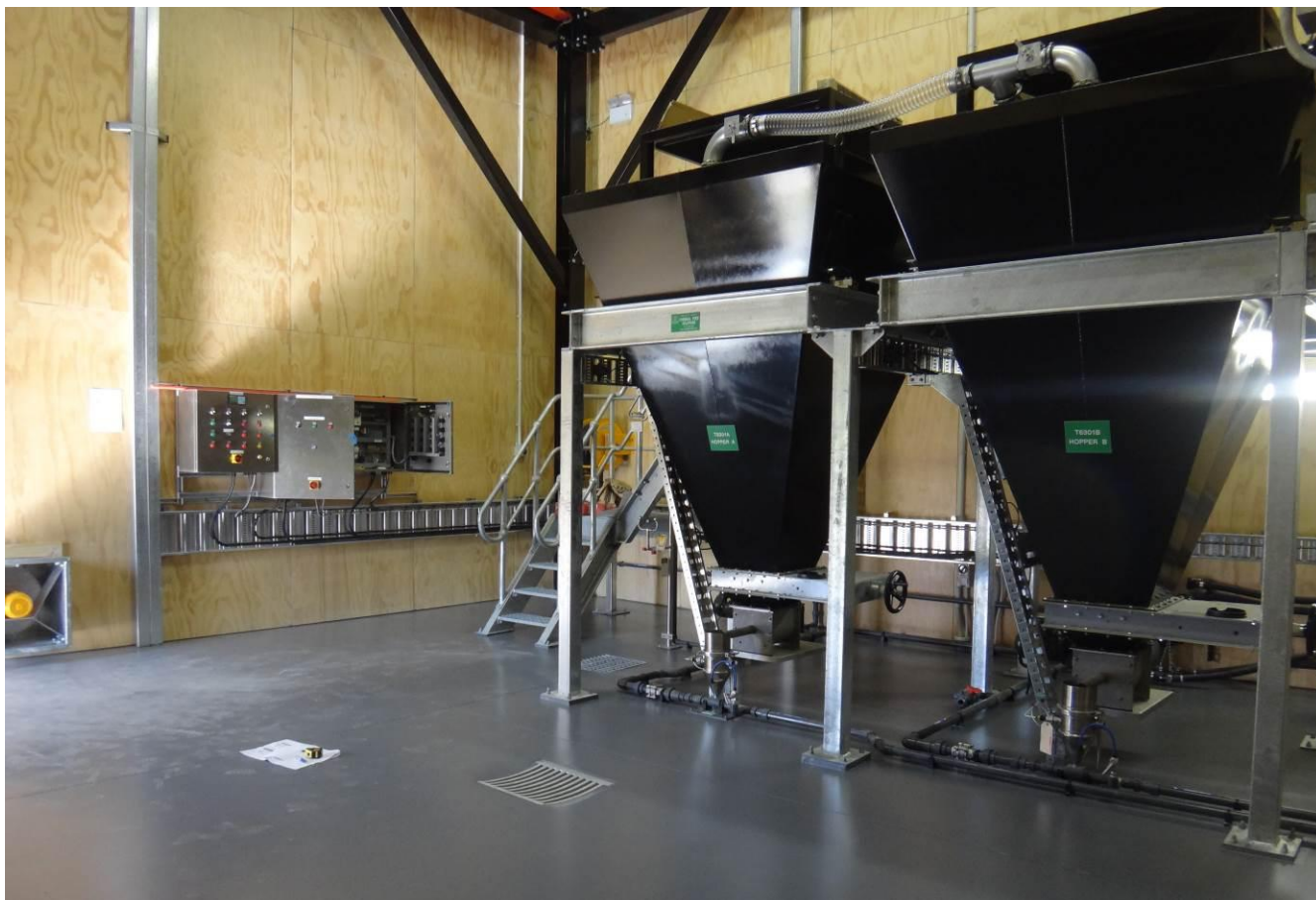
Photograph 7: Upgraded Powdered Activated Carbon Dosing System
