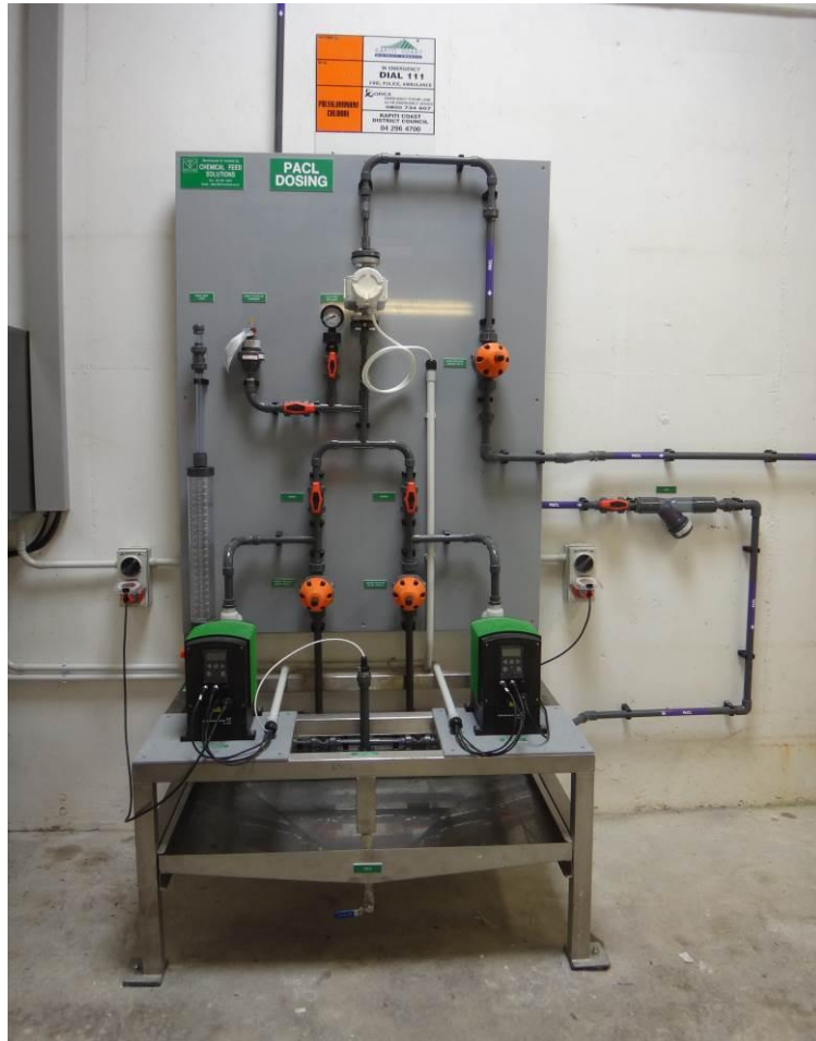
Photograph 6: Upgraded Poly Aluminum Chloride Dosing System
