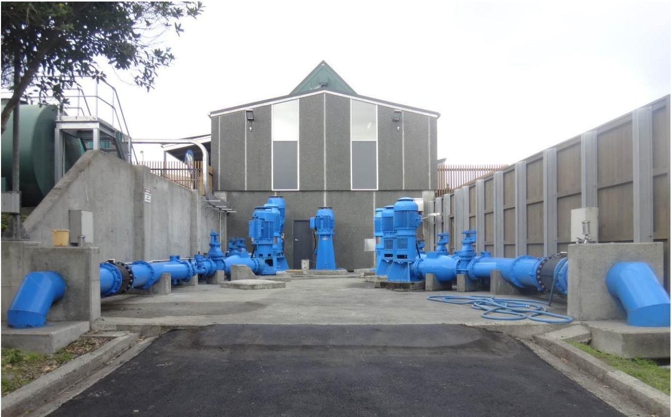
Photograph 9: Upgraded Treated Water Pump Station
