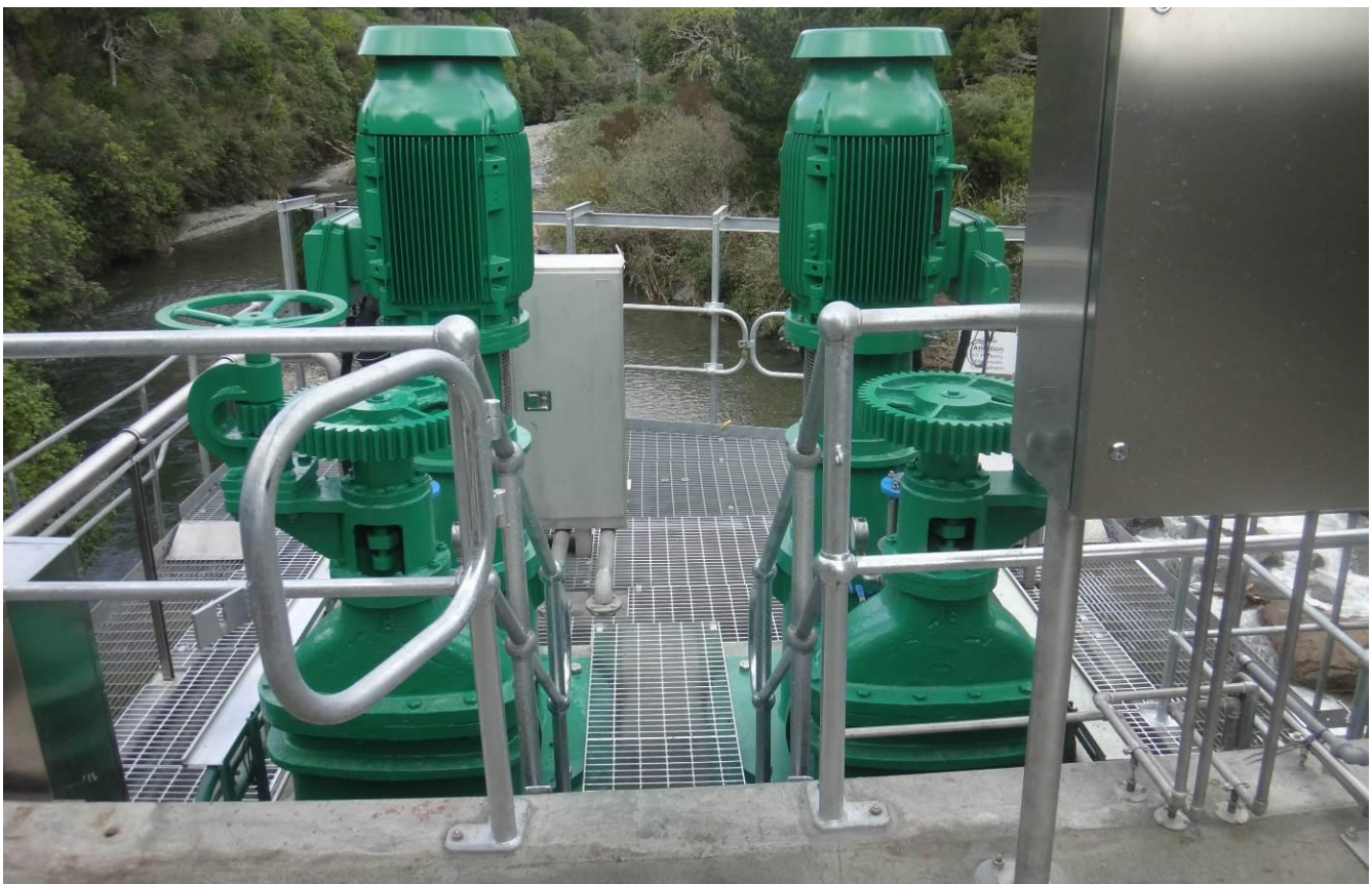
Photograph 5: Upgraded Raw Water Pumping Station
