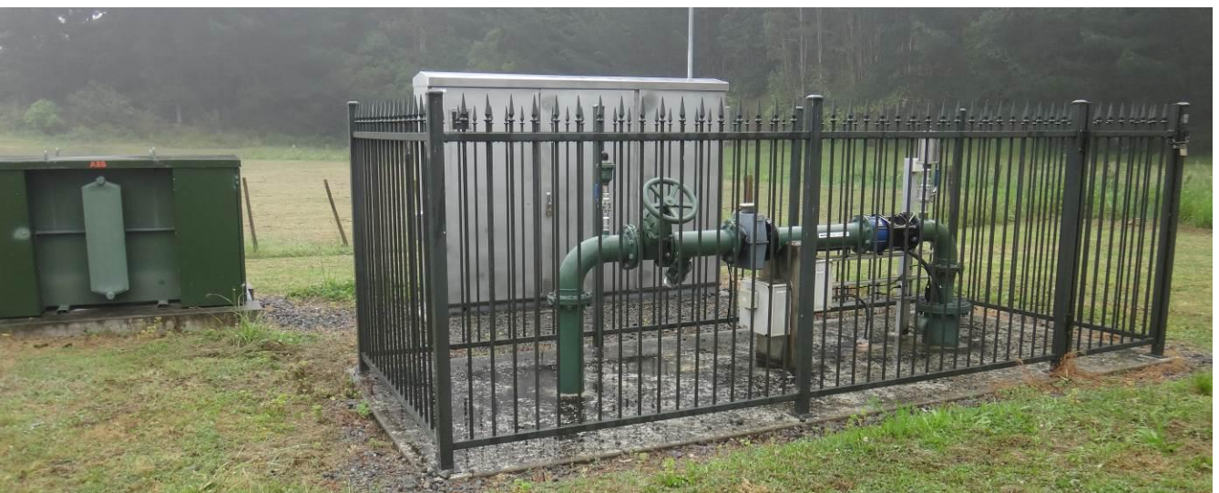
Photograph 2: Kb4 Bore Headworks on the Waikanae Borefield. Completed July 2005
