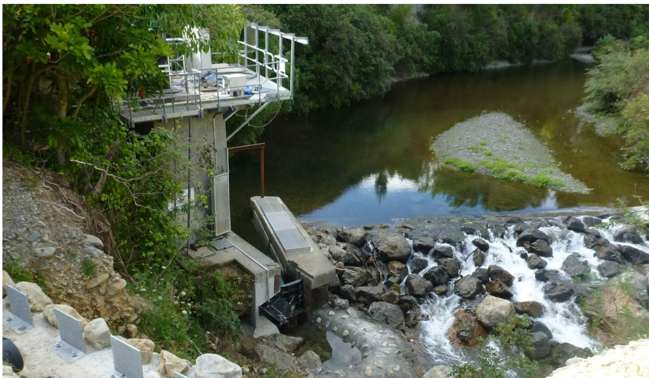
Photograph 4: Upgraded Raw Water Intake
