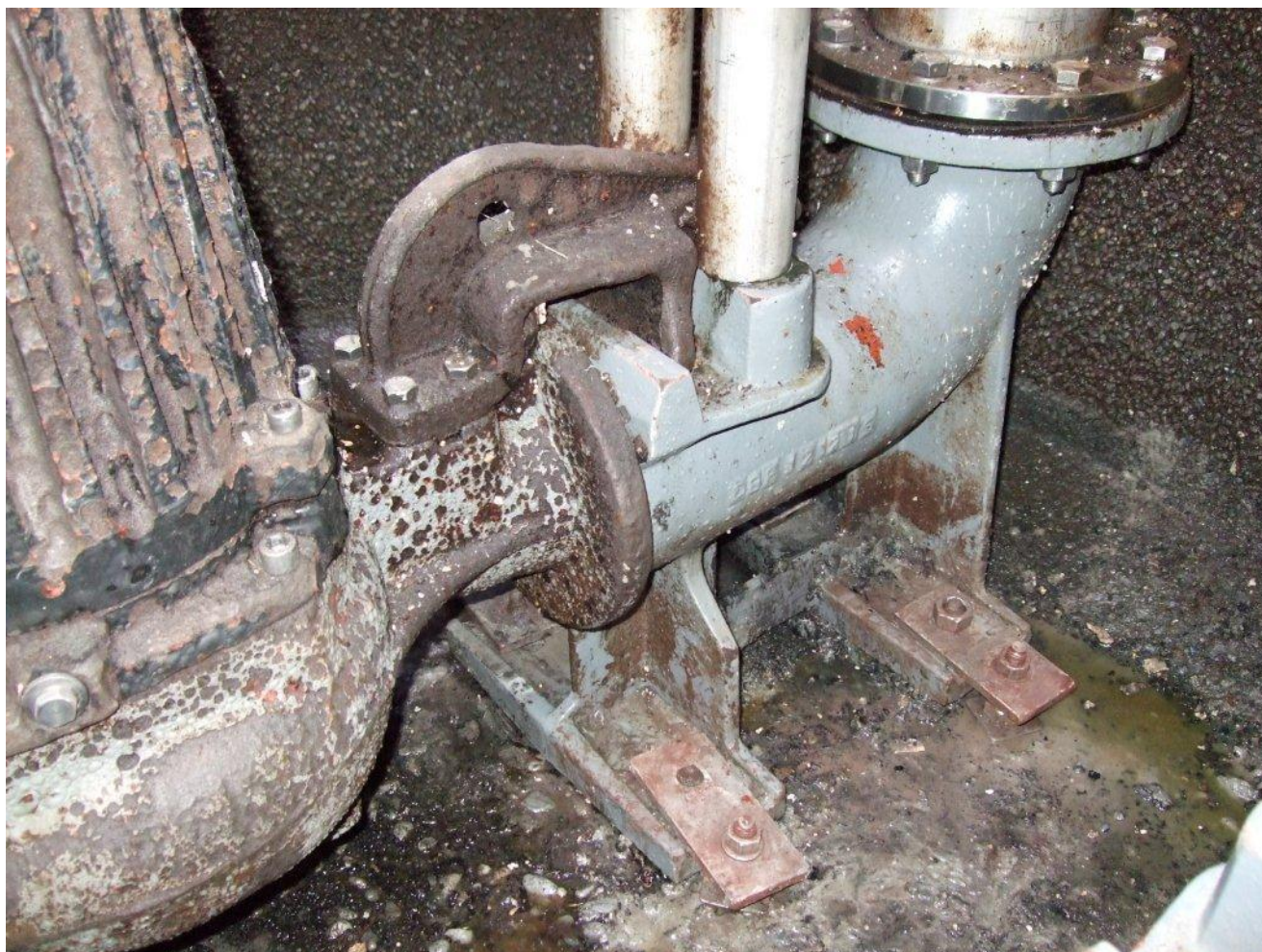
Photograph 1: Corrosion of pump and concrete wet well at the nearby Vernon Street South Pump Station
