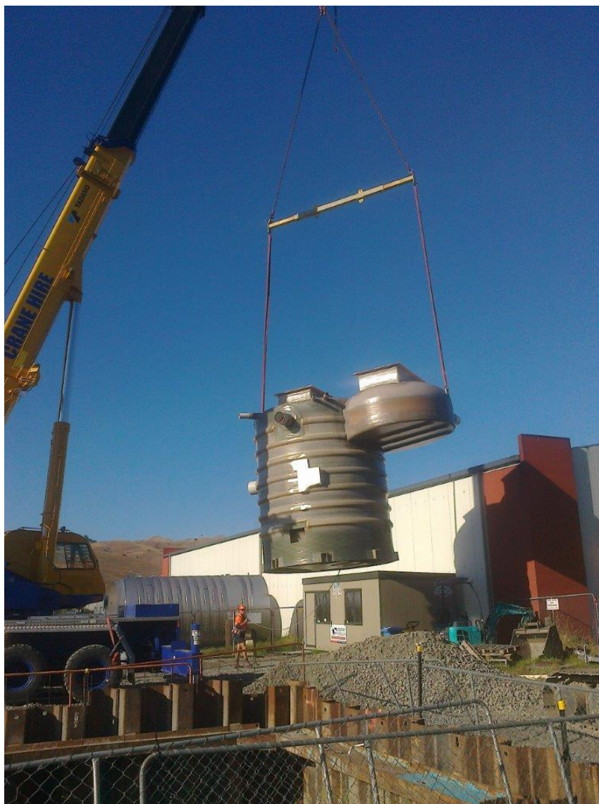
Photograph 2: The wet well and conjoined valve chamber being off-loaded from the low-loader vehicle onto the prepared base at Vernon Street Pump Station, Blenheim
