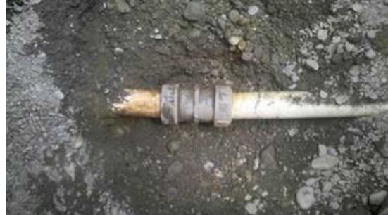
Figure 4. Leaking PE or PP bodied compression fitting on PVC pipe, Masterton. (Citycare).
