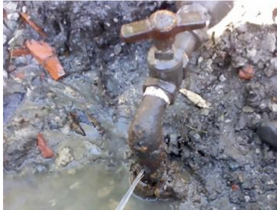
Figure 5. Perforated copper pipe leaking next to stop tap. Citycare.
