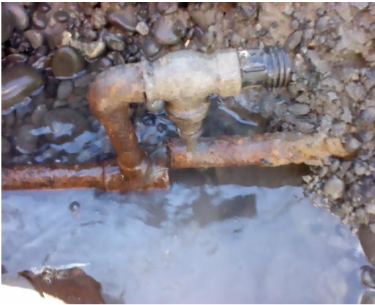
Figure 1. Complex geometry and mixed materials (Citycare). The low image quality is due to use of a camera phone.
