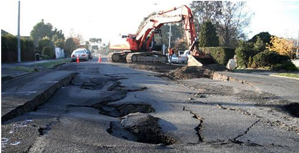
Photograph 12: Woodham Road Trunk Main Failure
