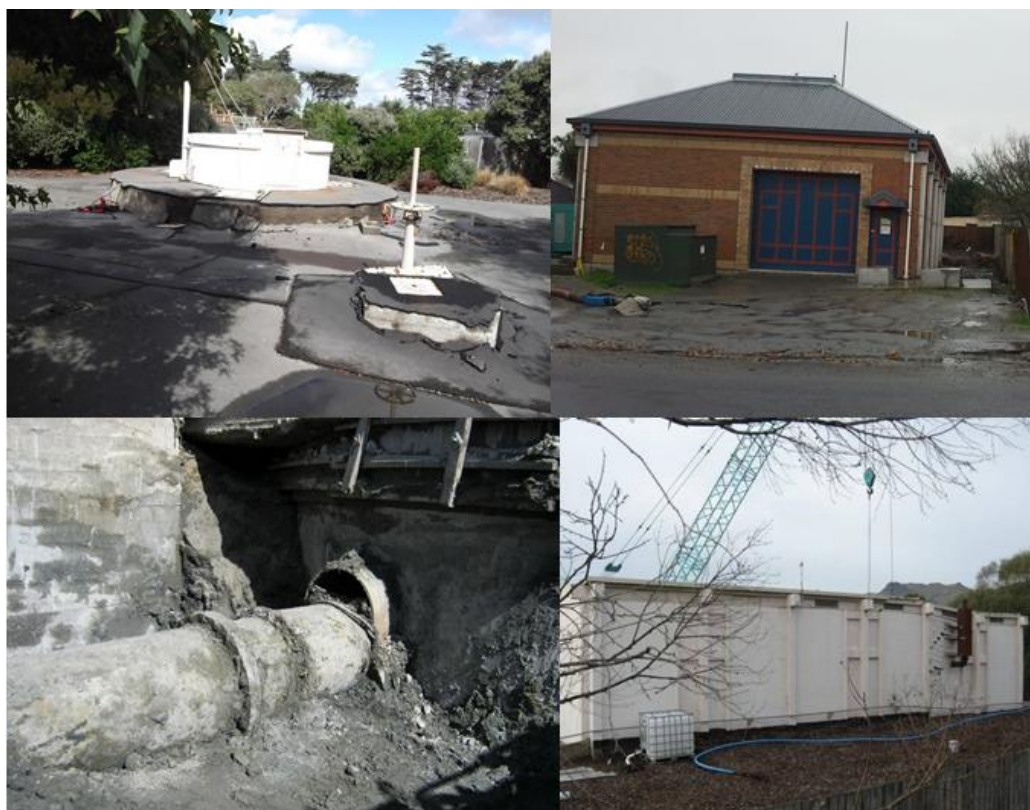
Photograph 9: Pump Station Earthquake Damage
