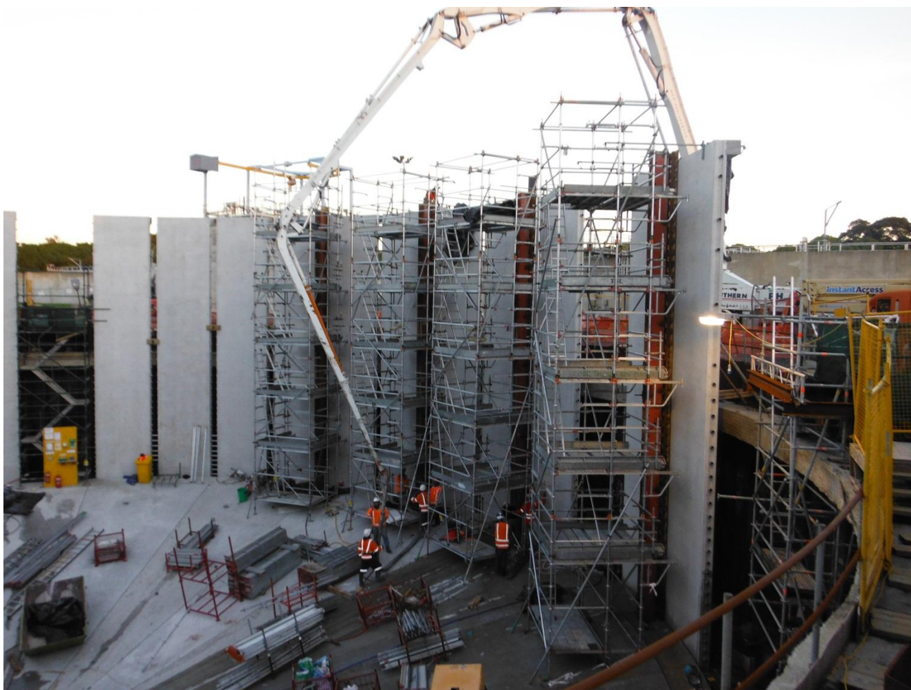
Figure 3 - Wall Stitch Joint Formwork and Concrete Placement. Note: Concrete Enters Near the Stitch Bottom
