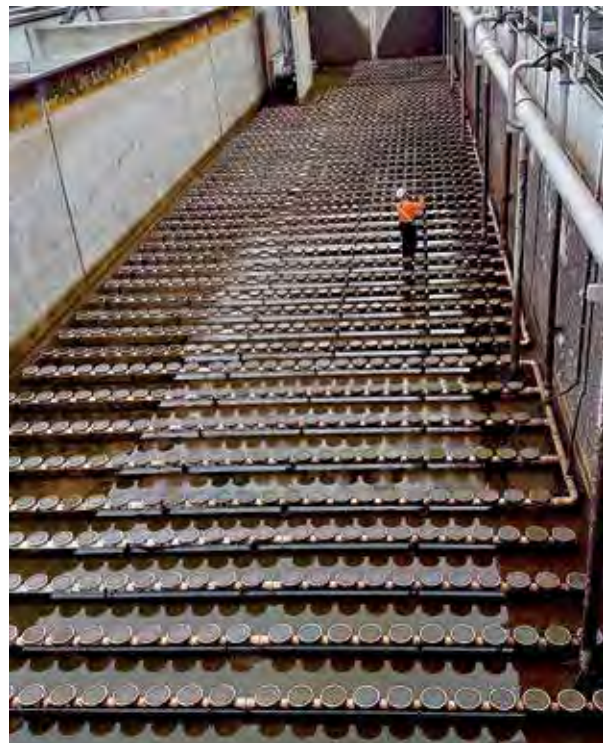
Fitter in basin, Wastewater Treatment Plant Pukete, Hamilton, Martin Scott.
