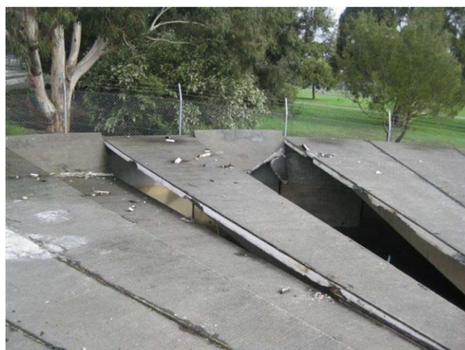
Photograph 3: Damaged Denton Park reservoir roof in September 2010 Christchurch earthquake
