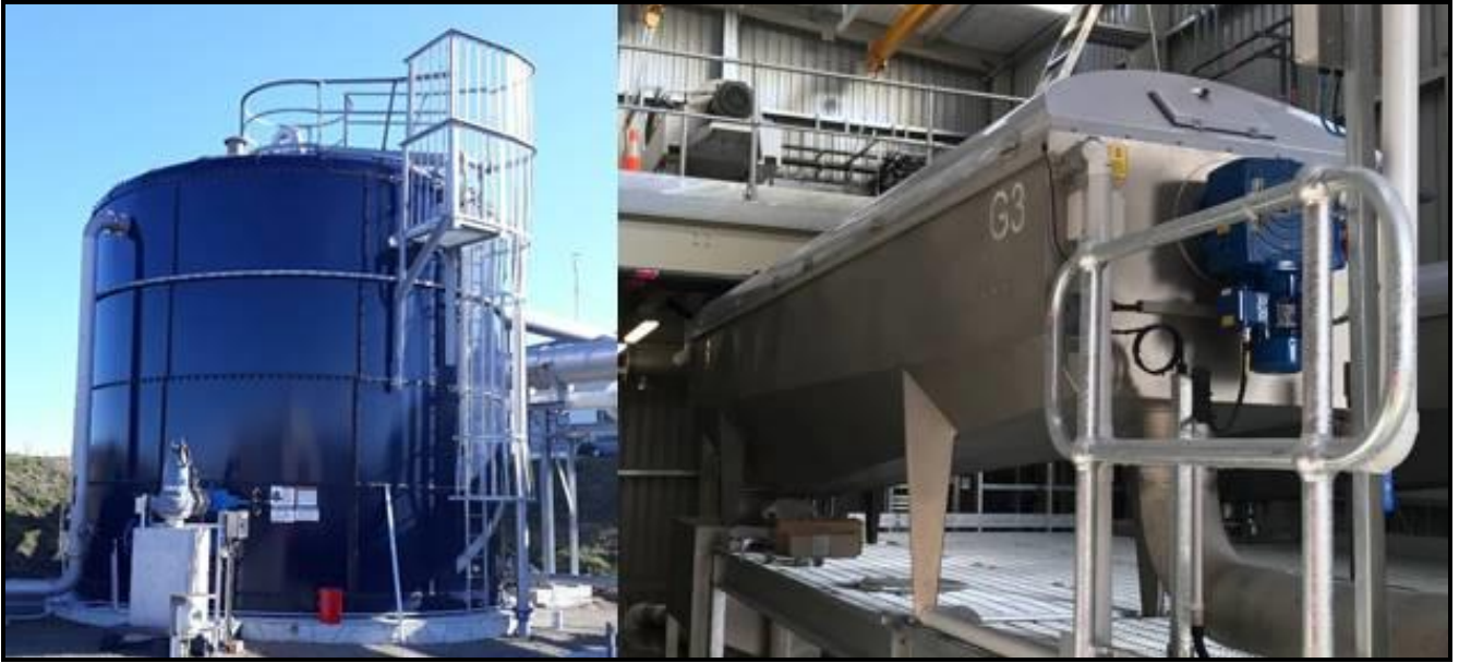
Photograph 11/12: Decanter Centrifuges (left), Dewatered Sludge Silo (right)
