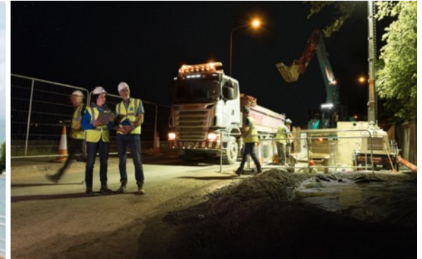
Cork Harbour Main Drainage Scheme
