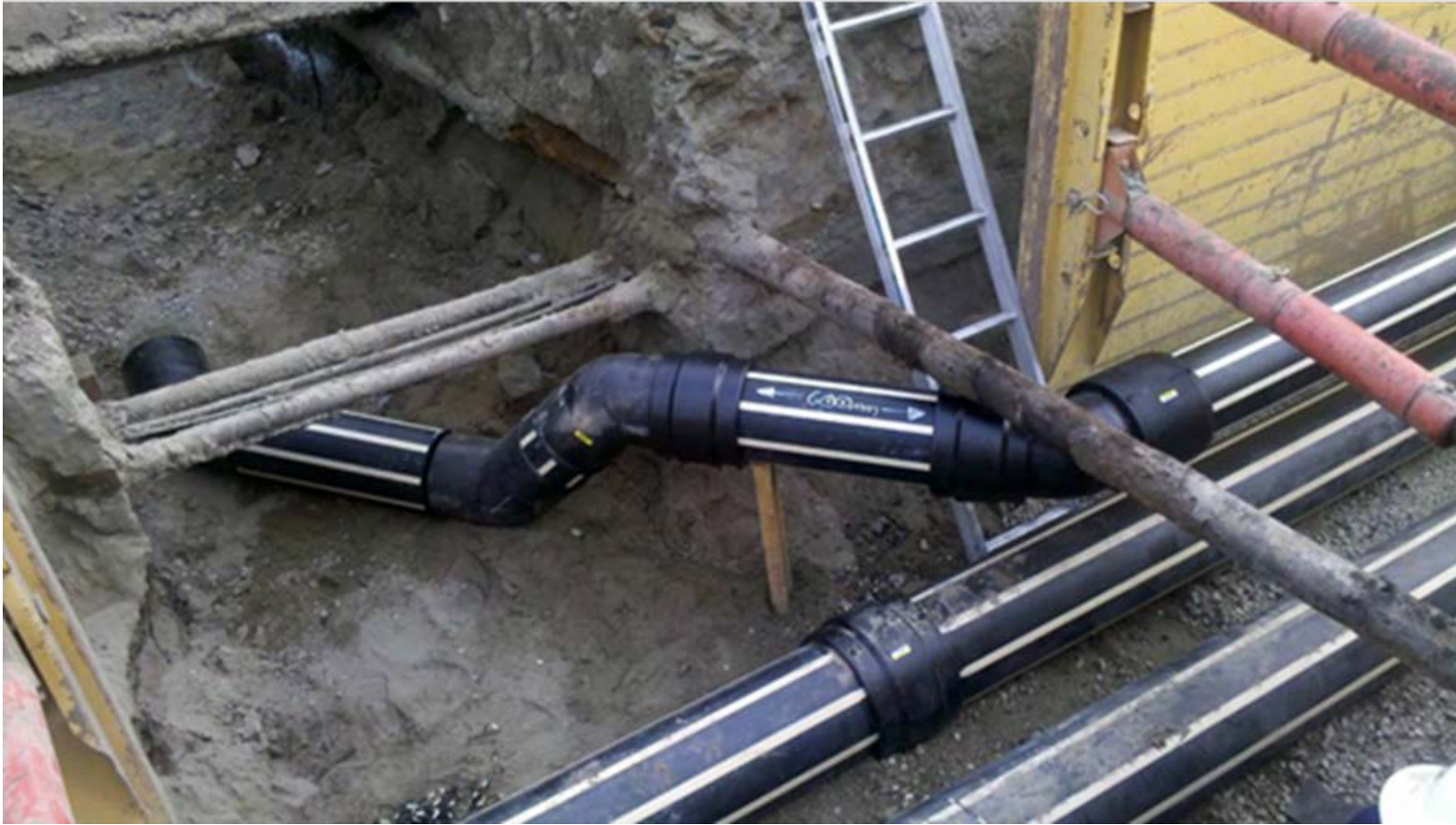
Vacuum Main Installation
