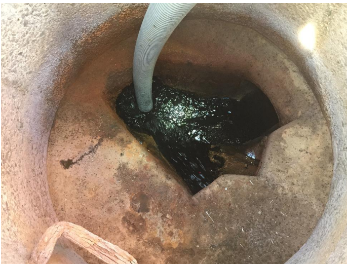
Photograph 4: Ice and sludge arriving at the discharge manhole.
