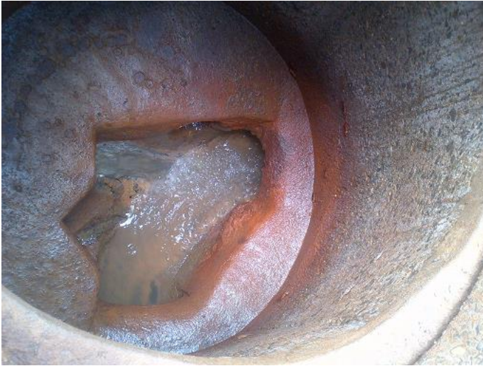
Photograph 4: Clean ice at the discharge manhole.
