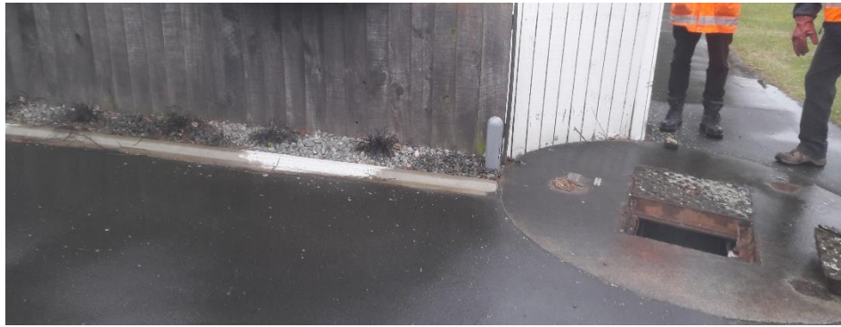
Figure 2: Example of a well head with surface water drainage paths into it
