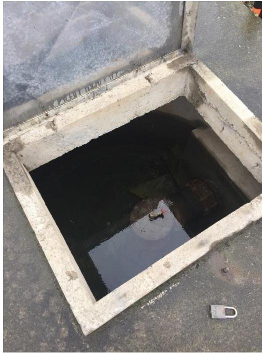
Figure 1: Example of a well head chamber filled with water
