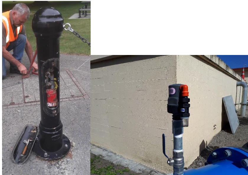
Figure 4: Examples of an air vent outside of a well head
