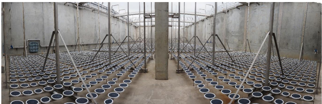
Photograph 2: Installed disc diffusers on removable grids
