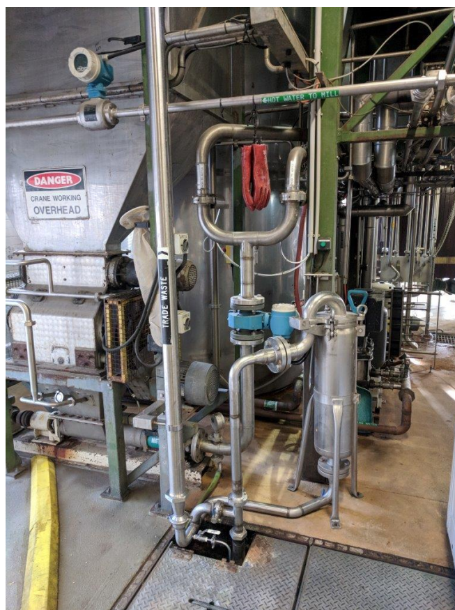
Photograph 1: Trade Waste sump and lead bag filter with steel mesh insert
