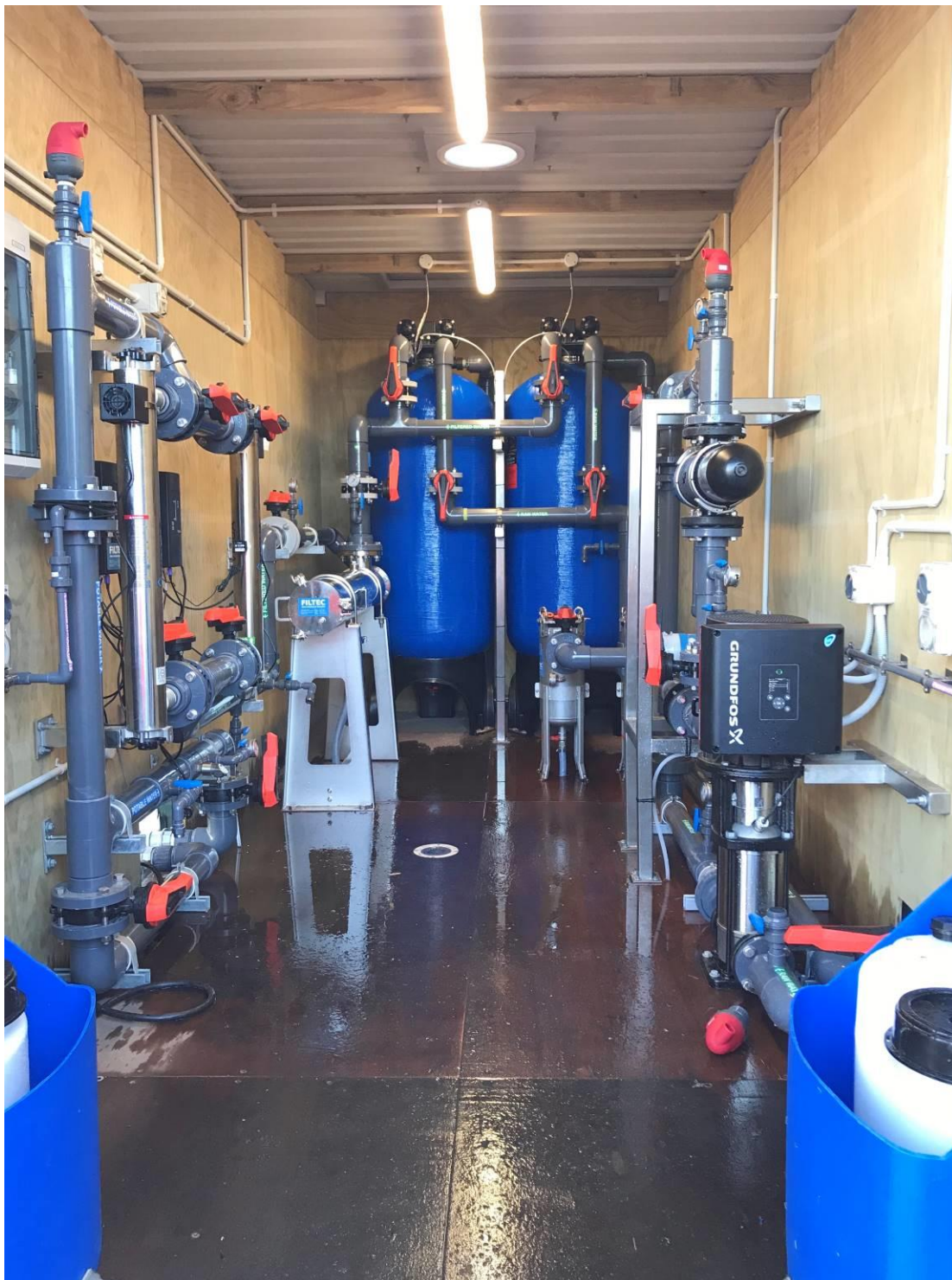
Figure 6 – Surface Water Treatment Station
