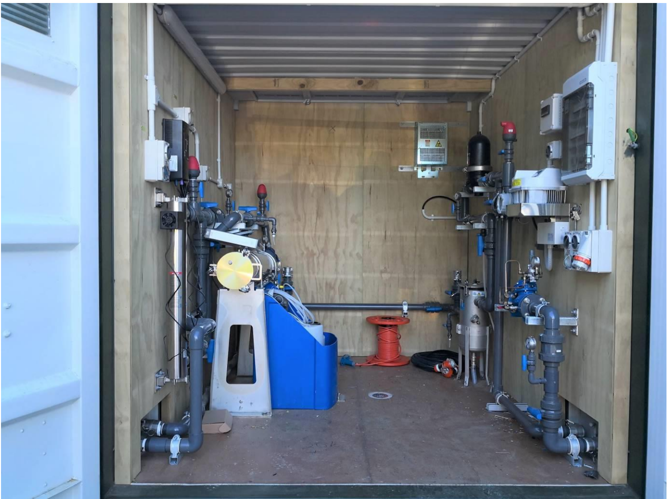
Figure 7 – Ground Water Treatment Station
