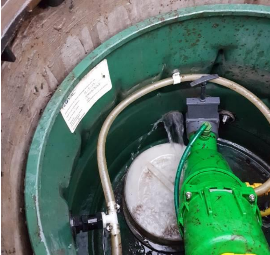
Figure 8 Infiltration Through a Duct into the top of the VSS Collection Chamber
