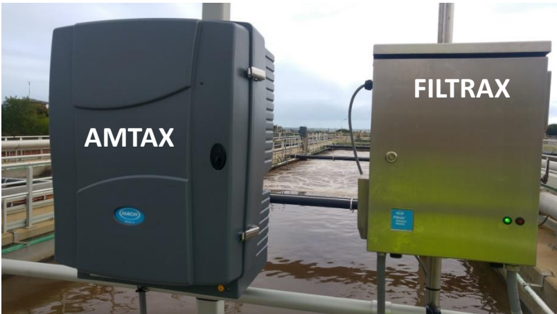
Figure 5: AMTAX and FILTRAX units
