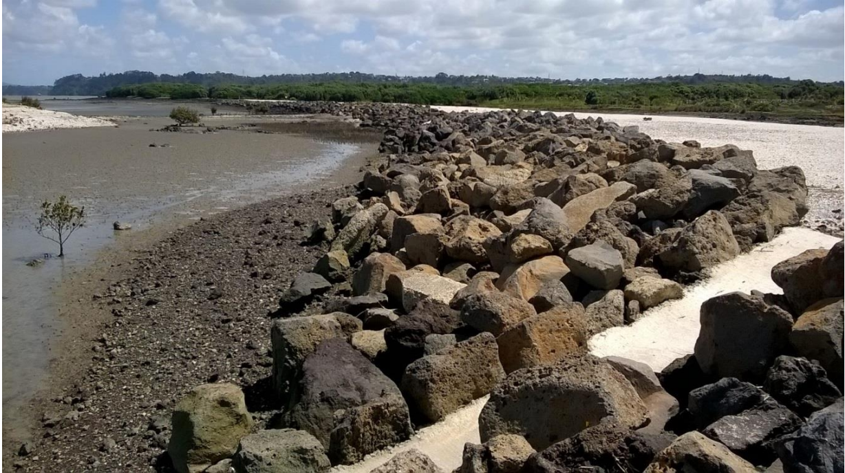
Photograph 2 'Long Island' bird roost with the newly installed riprap wall and in the foreground one of the 12 NZ dotterel chick pathways laid at an angle to the prevailing wind & wave direction.
