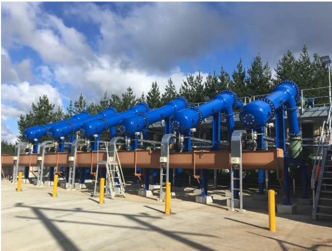
Photograph 7: LAKOS sand hydrocyclone units and sand collection trough
