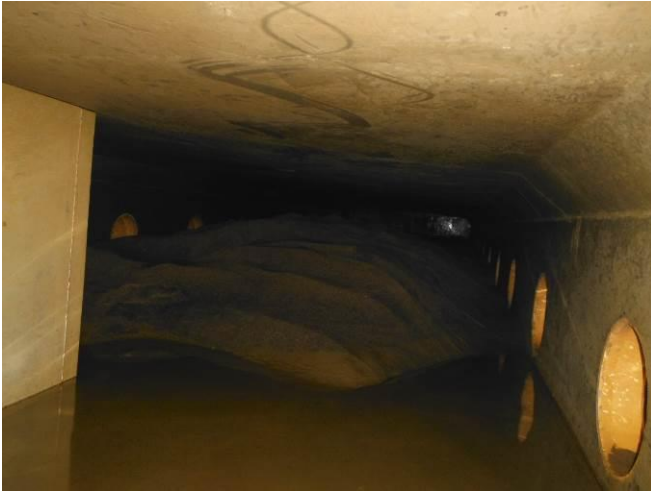
Photograph 5: Sand accumulation in the clarifier inlet channel
