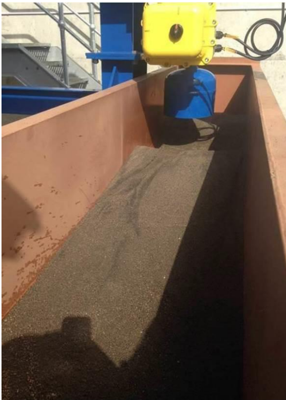
Photograph 9: Sand accumulation with the diffusers on the purge valve outlets
