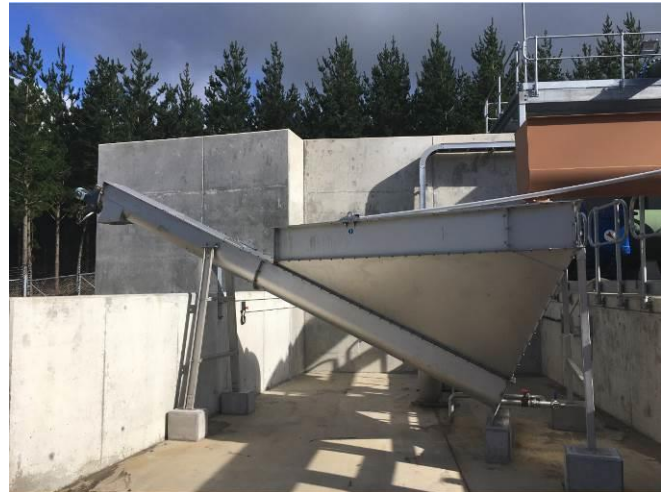
Photograph 8: Sand collection trough feeding into the top of the grit classifier
