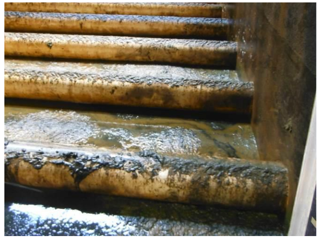
Photograph 6: Sand accumulation in the clarifier base
