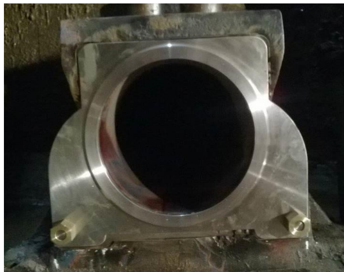
Photograph 4: Pedestal face plate mounted on each pump to counter sand abrasion
