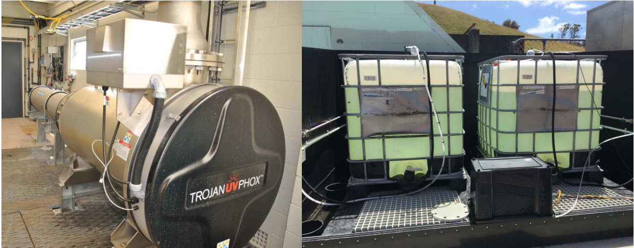
Photograph 3: Waihi UV reactor (left) and hydrogen peroxide IBC store (right)
