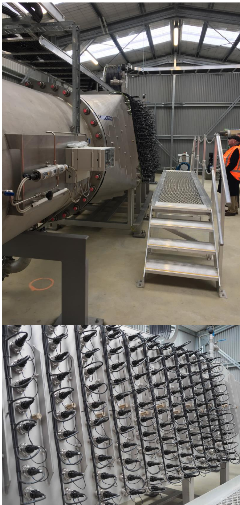
Photograph 1: Branxholme WTP UV reactor
