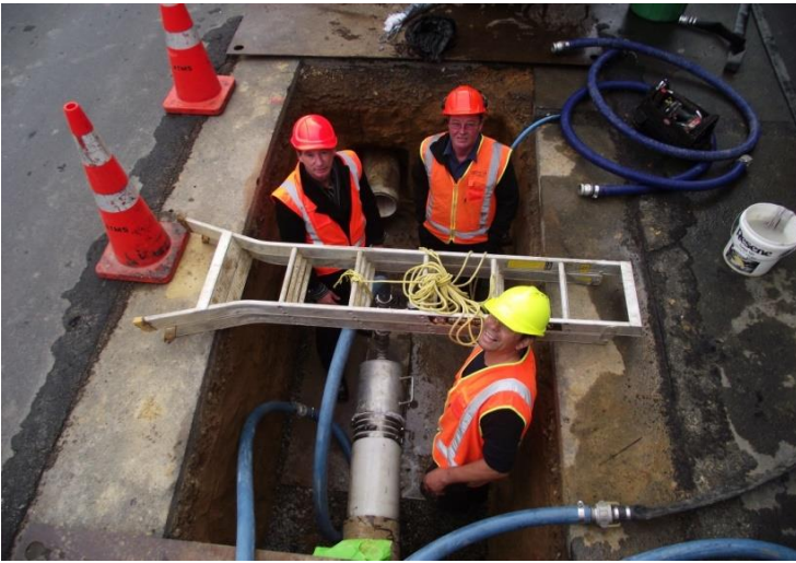
Relining Pit: 'Pig Catcher' in action, catching the forming swabs as they are propelled through the line during the forming and curing process
