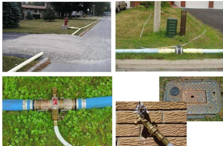
Figure 2: Temporary water supply
