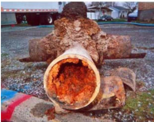
Figure 9: Water Main Before Cleaning
