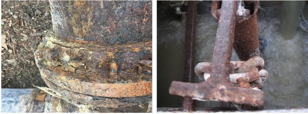
Figure 4: Examples of asset condition. Corrosion on flange bolts of riser (left) and rail bracket coming away from wall (right)
