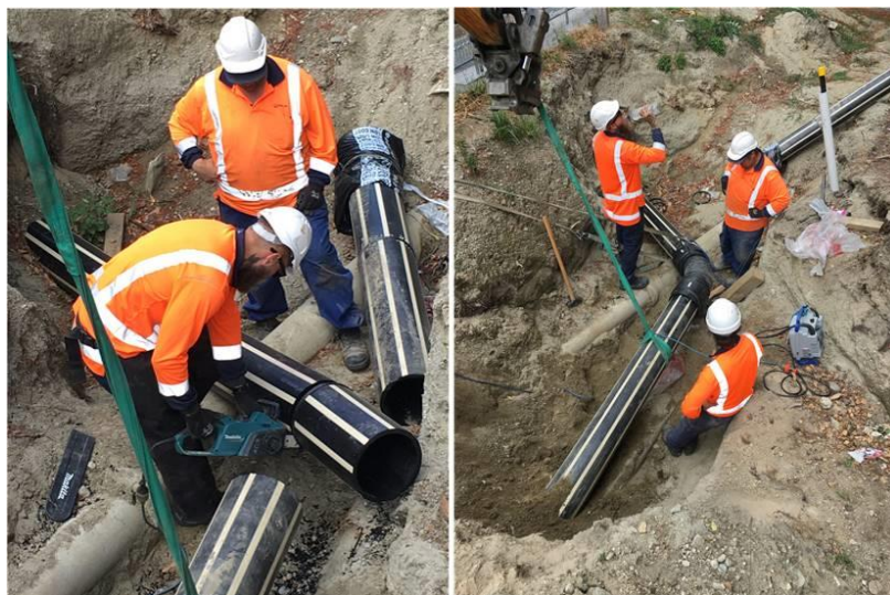
Figure 10: Having the right fitting in the right place, the result of careful planning and careful measurement
