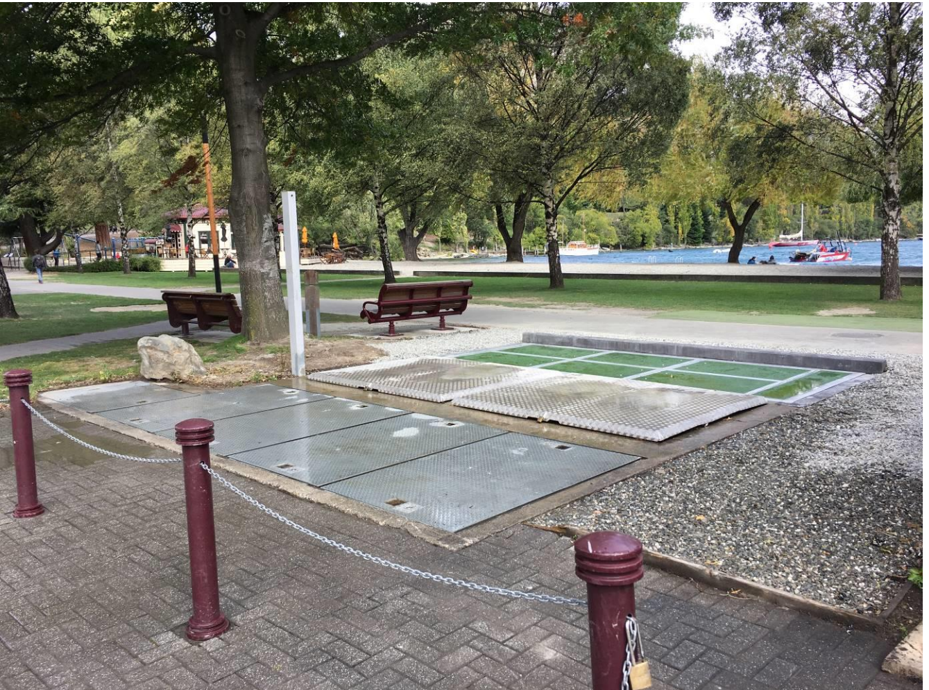
Figure 13: On completion, hardly a trace that a major, complex project on critical infrastructure has been delivered.
