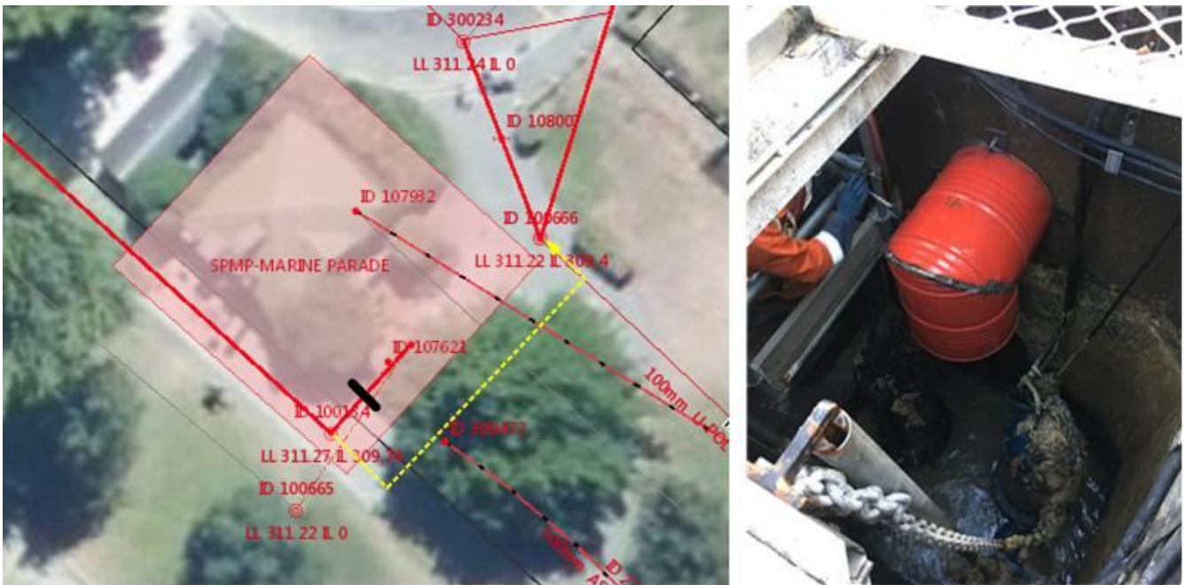
Figure 5: During a low-flow period, an inflatable bung was inserted into the pipe from Fernhill (at the black line) and a pump-around set-up (yellow) to enable fitting of a temporary baffle to protect workers in the well (right photo).
