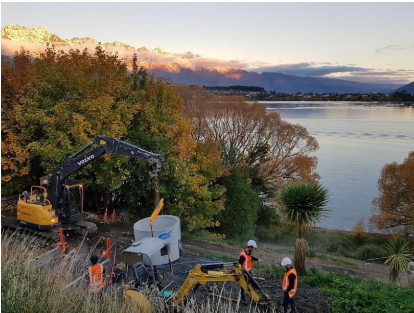
Figure 11: No margin for error working on live sewer assets this close to the lake
