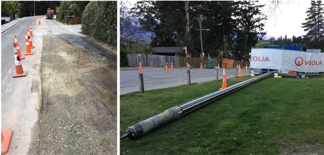
Figure 8: Detailed investigation and measurement identified a missing section in the abandoned main. Replacement duct (left) was laid within a short space of time, minimizing traffic restrictions on Park St, allowing pull pit and welding to be established off the carriageway (right).
