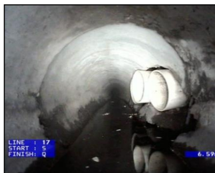
Picture 5: Intruding lateral junctions
