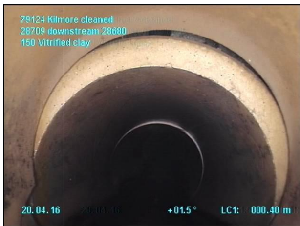
Picture 7: Displaced or dropped joint
