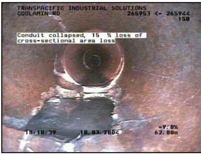
Picture 1: Sewer with missing section
