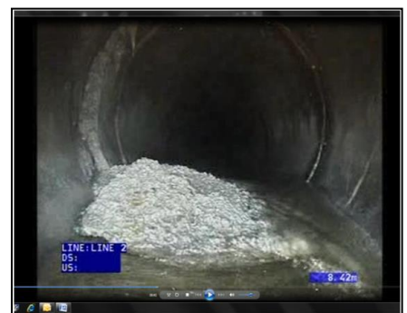
Picture 6: Debris, possibly silt, rubble or concrete
