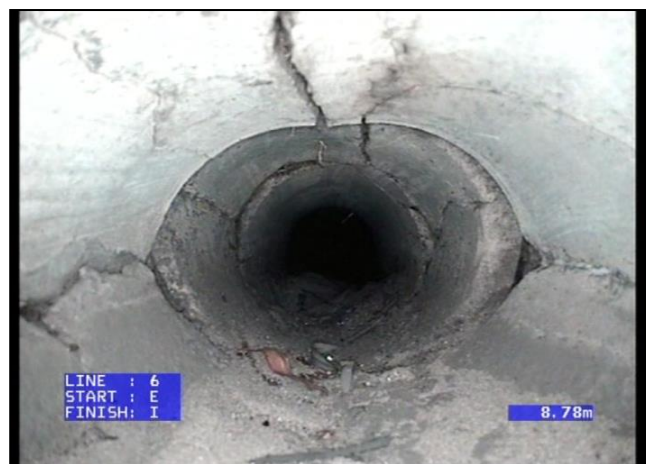
Picture 8: Deformed pipe, partial collapse
