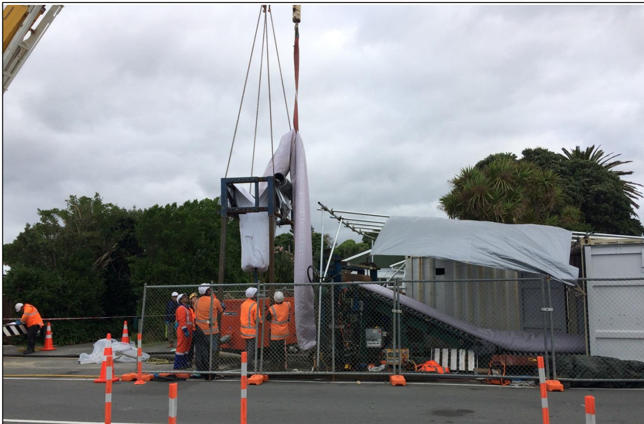
Figure 7: Liner being raised over the insertion manhole for inversion under head pressure
