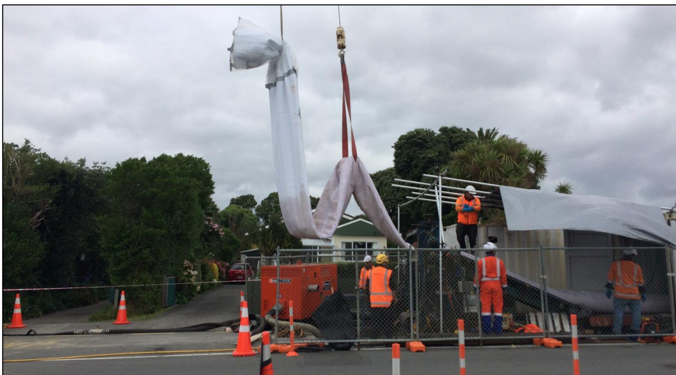
Figure 8: Liner being raised over the insertion manhole for inversion under head pressure.
