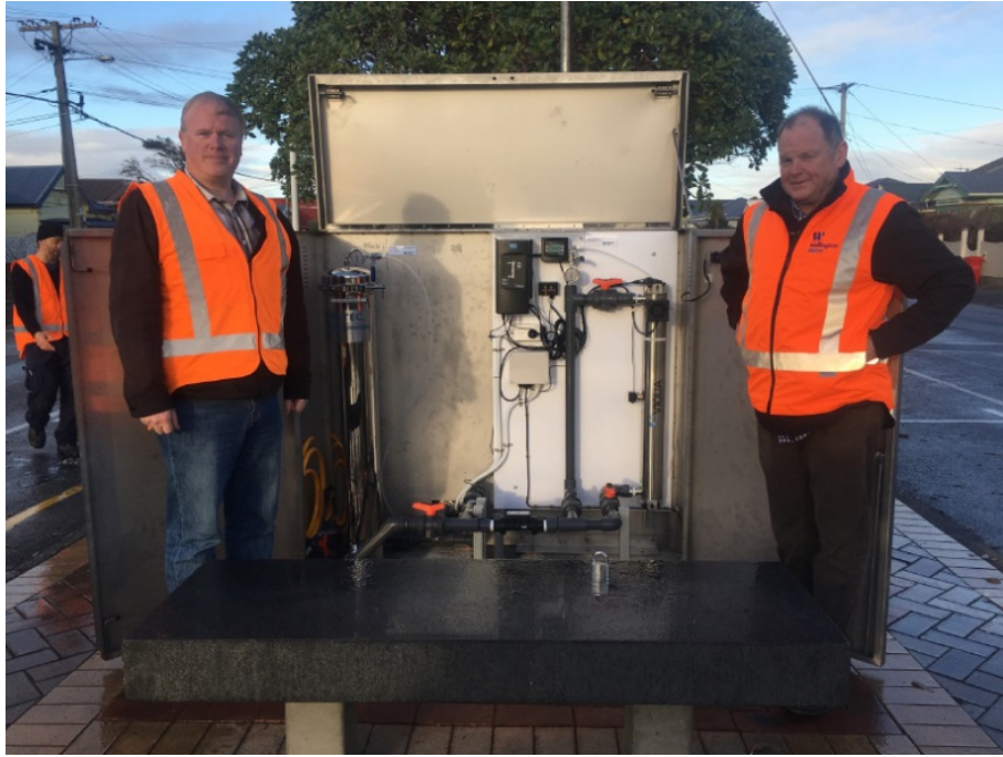
Figure 10 – Package Treatment (UV and filtration) installed at Buick Street
