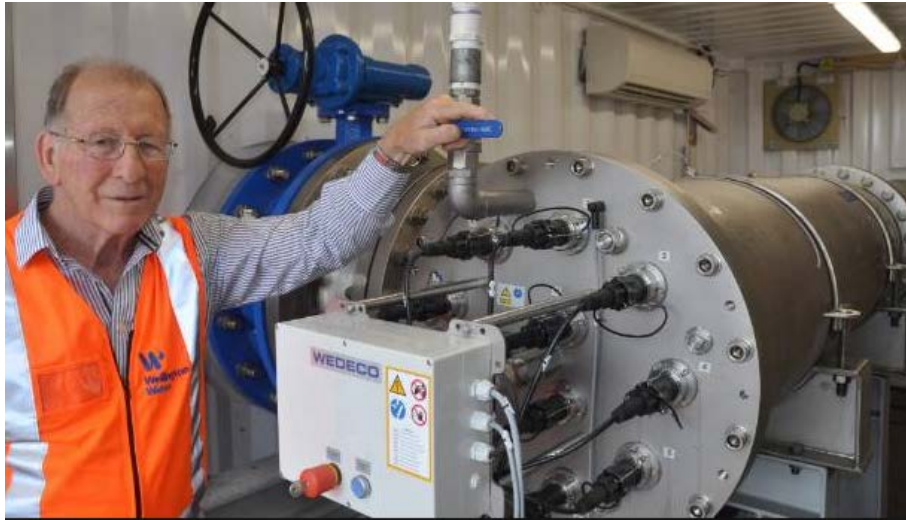
Figure 12 – Chris Laidlow, GWRC Chairman, at the Waterloo WTP UV plant
