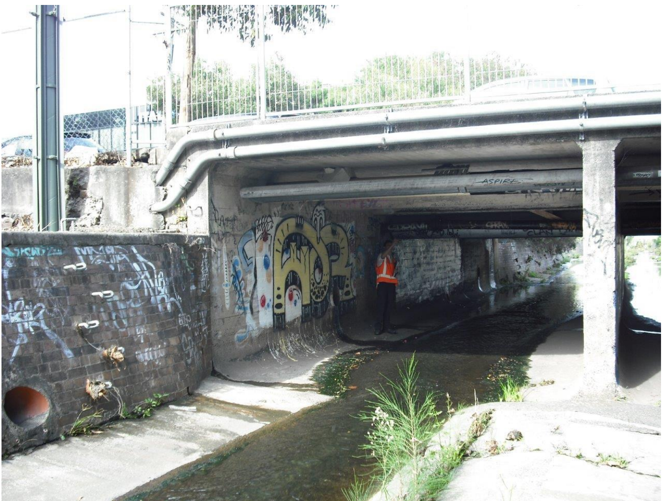
Photograph 4: Existing Huntley St culverts showing the many intruding services
