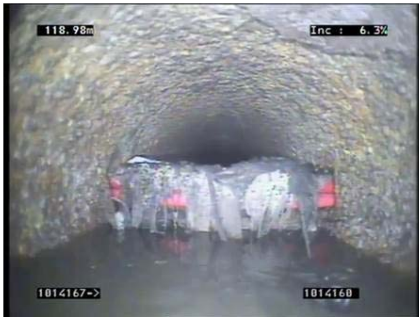
Photograph 2: 11 kV cable ducts drilled through the Eastern Interceptor
