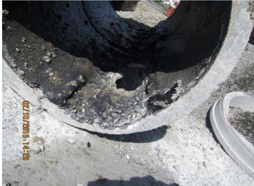
Photograph 1: Section through a failed concrete pipe from Victoria Street
