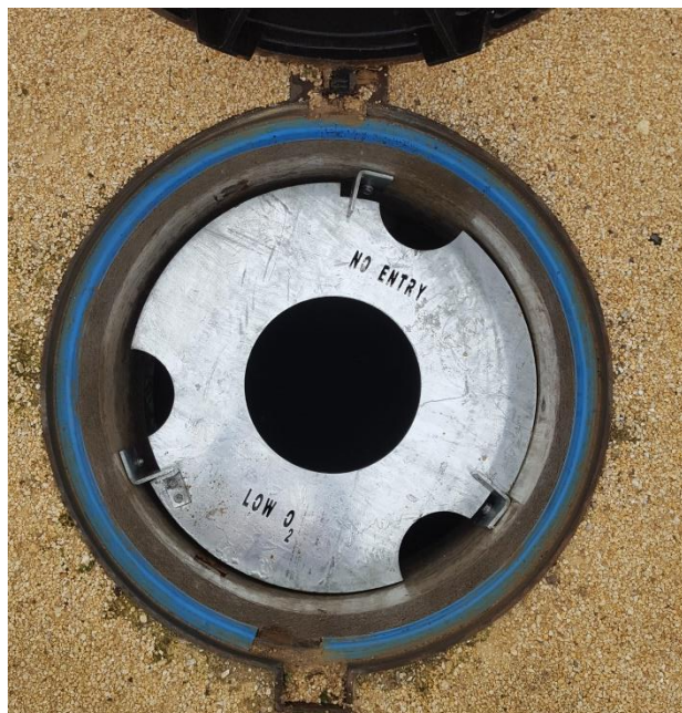
Figure 13: Soakage Chamber Access Lid
