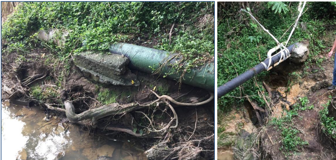
Photograph 2 & 3: Abutment being undermined. Undermined abutment with temporary support (Barnes, 2017)
