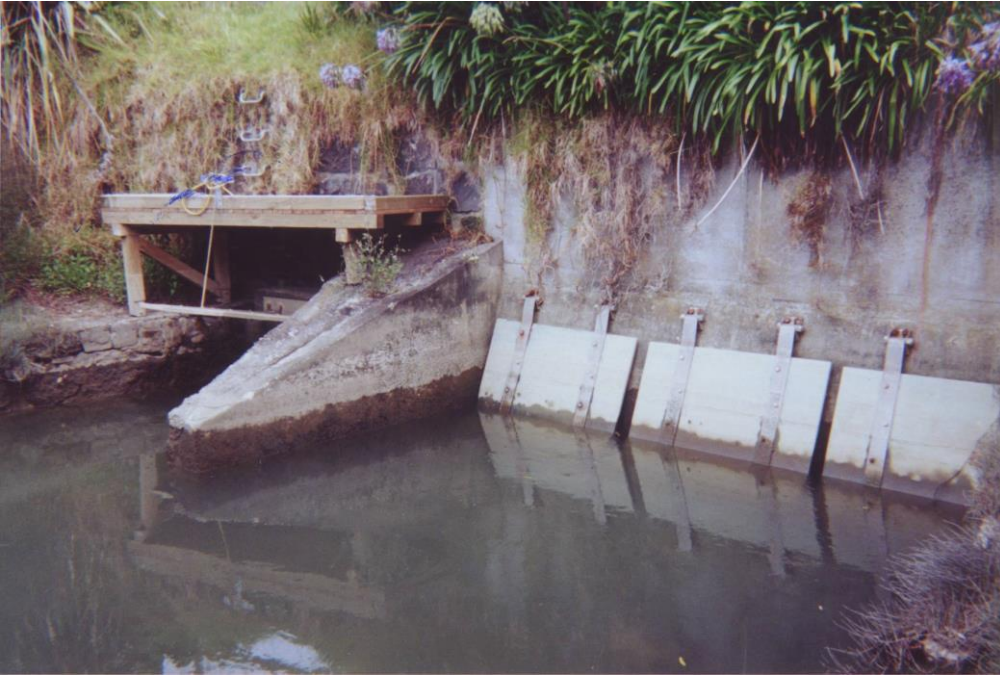
Fig 5 Tidal gates near Portland Road
