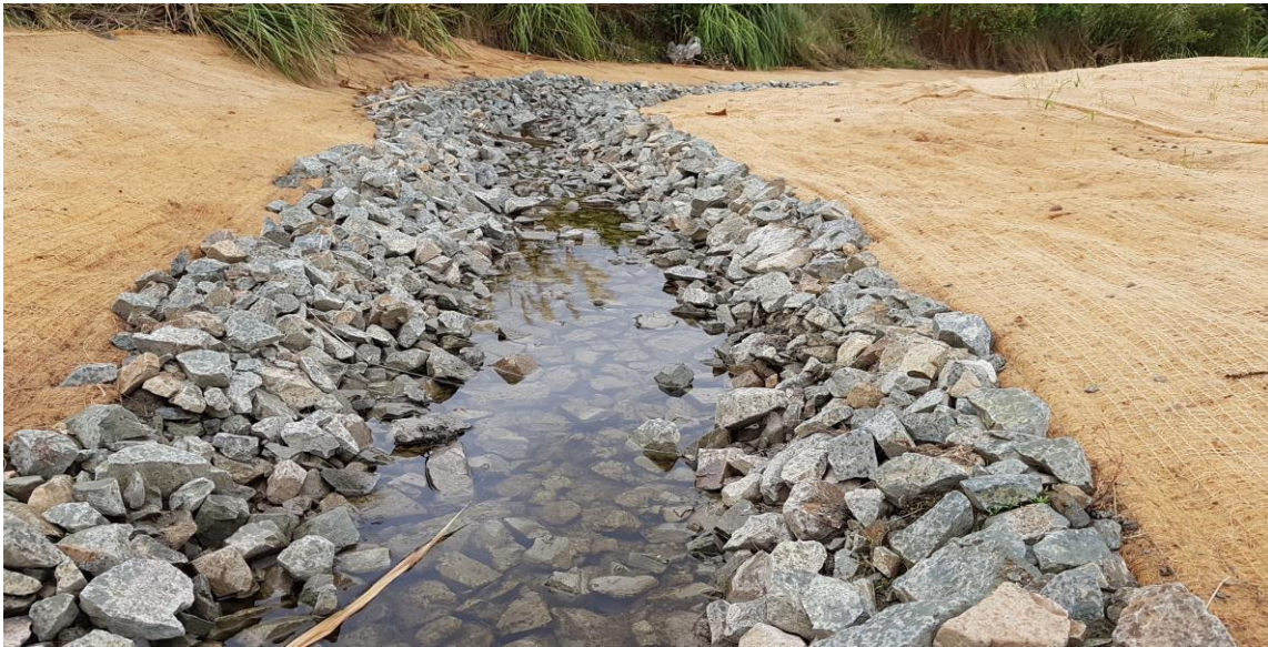
Photograph 3: Low-flow channel within the Cooks Lane reach of the Matuku Waterway currently under construction in January 2018.
