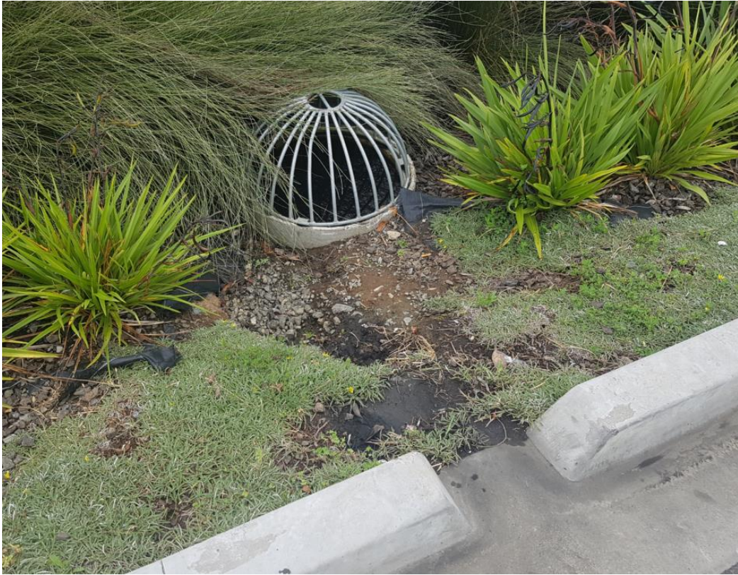
Figure 12: Erosion at raingarden inlet
