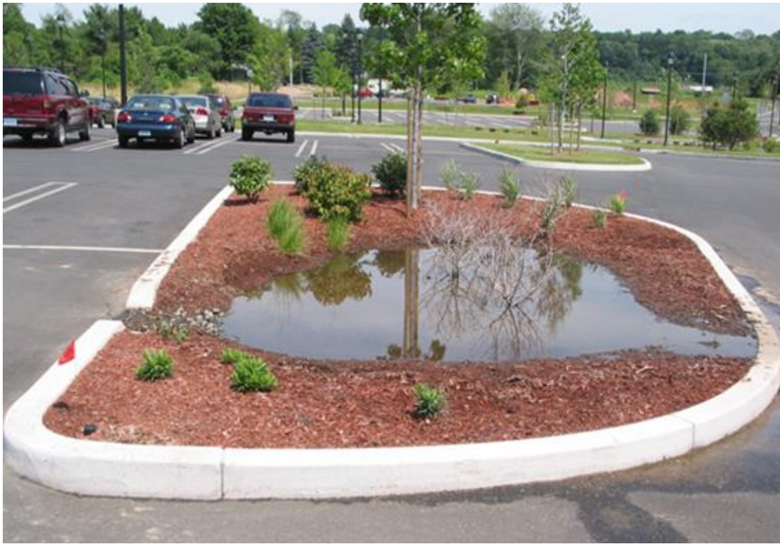
Figure 11: Overflow from Raingarden
