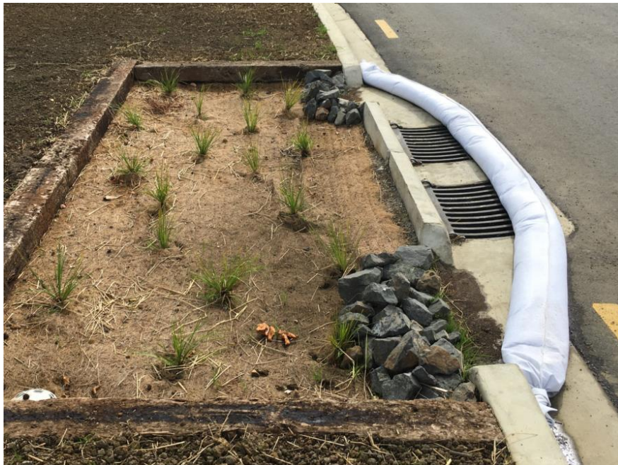
Figure 13: Accumulated sediment at raingarden inlet
