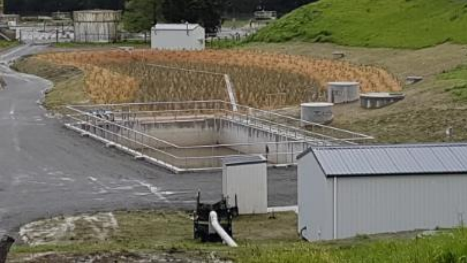
Figure 2: Overall view of first flush tank (centre) with swales (top) and monitoring sheds (bottom right, and top).
