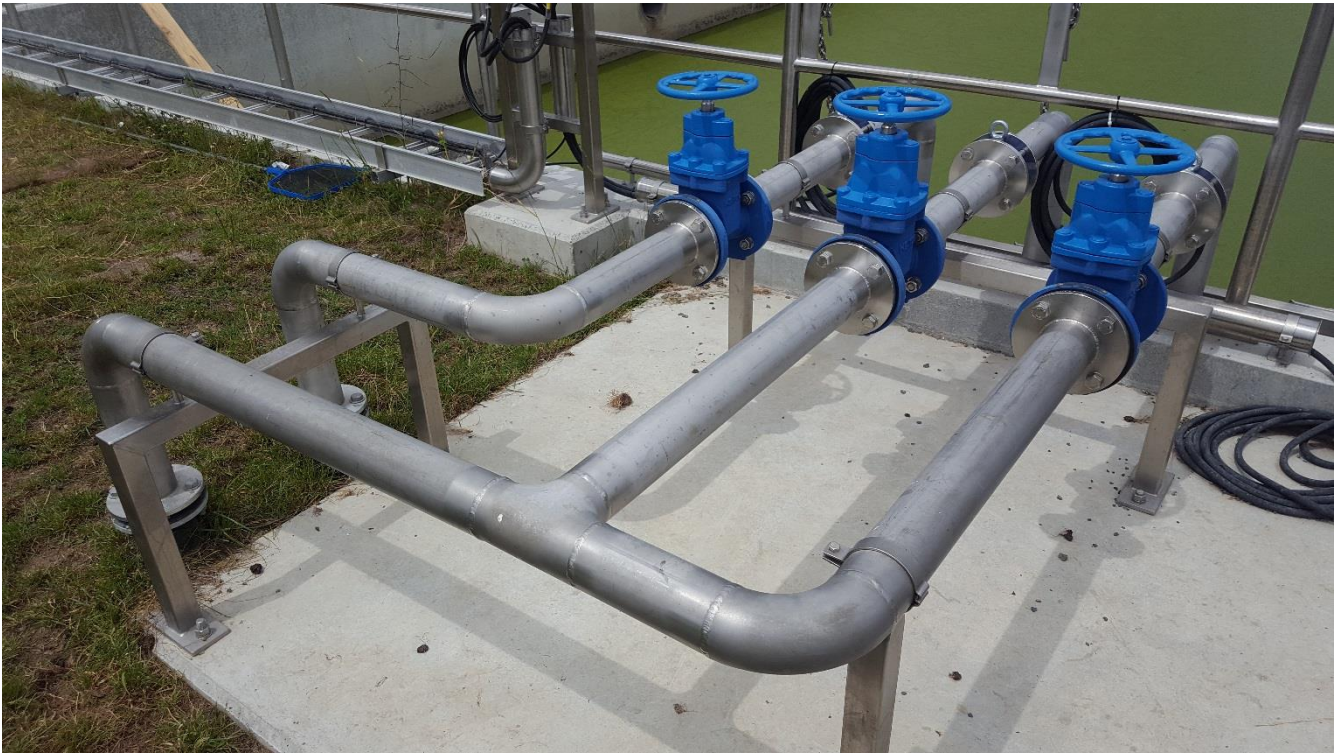
Figure 3: Pump station from first flush tank for transfer to wastewater or swales.
