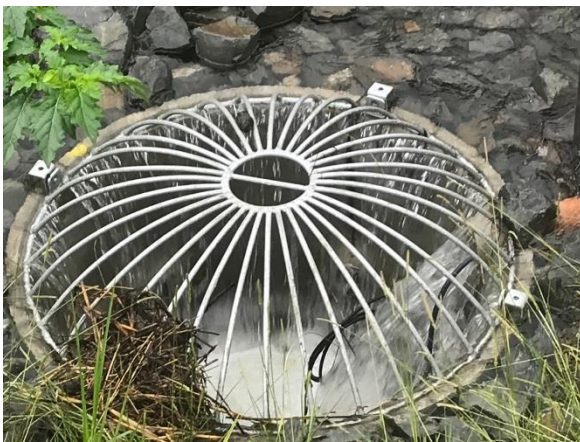
Figure 10: Swale discharge during heavy rain event.
