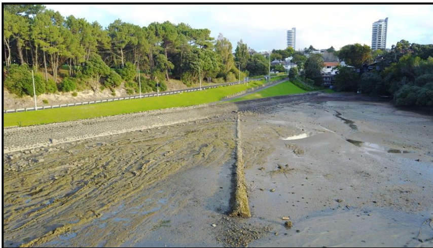
Photograph 3: Failed marine outfall at Masefield Beach
