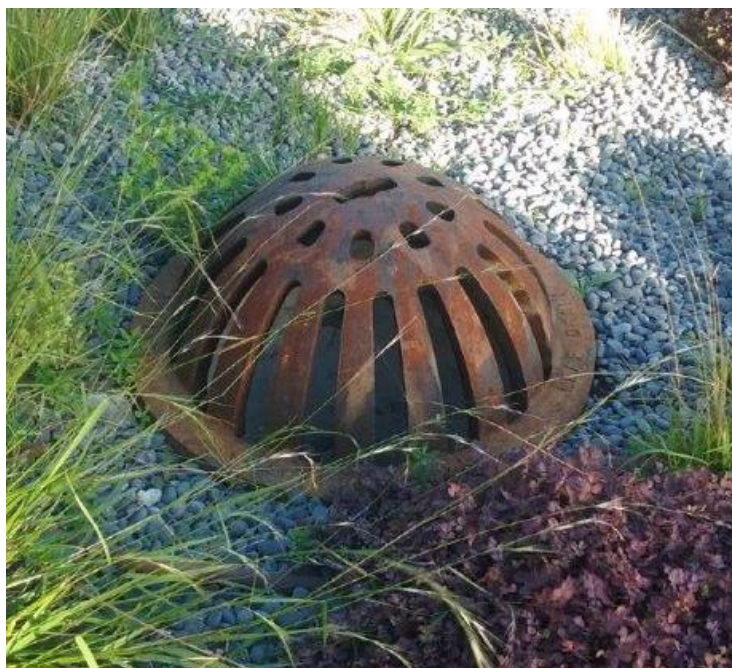
Figure 7: Dome sump inlet
