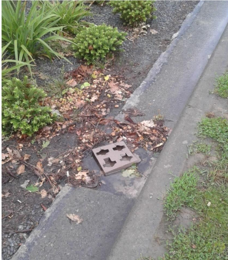
Figure 16: Litter partially blocking an inlet
