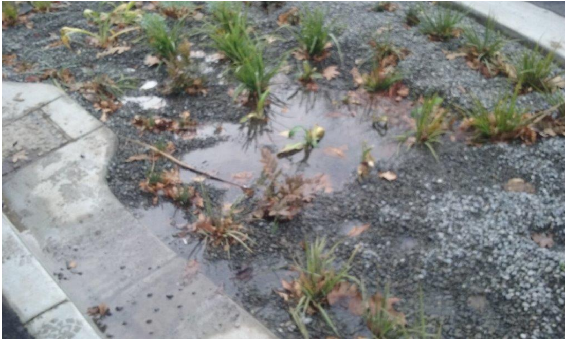
Figure 12: Depressions within a rain garden surface
