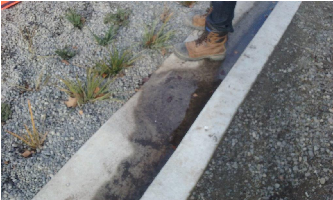
Figure 9: Poorly performing kerb inlet with noticeable ponding
