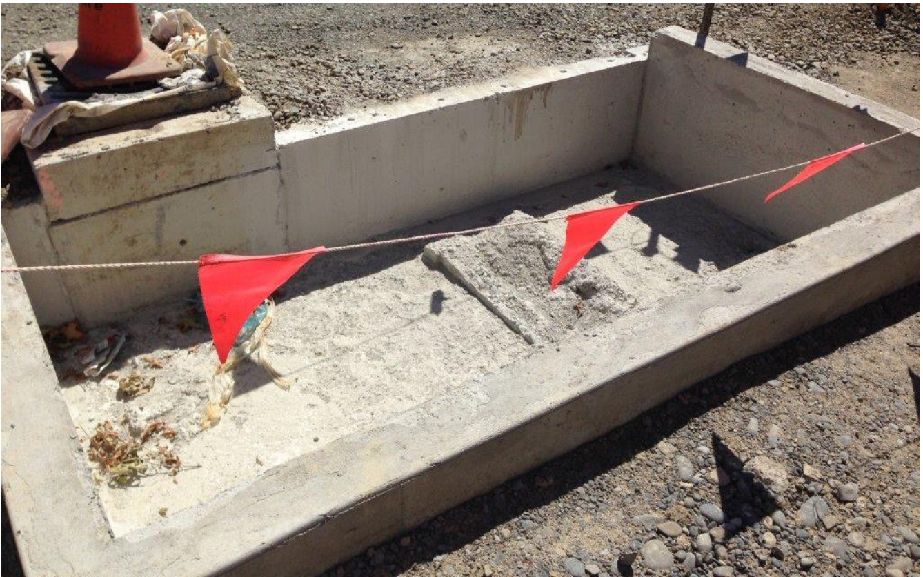
Figure 11: Concrete disposed of in base of rain garden
