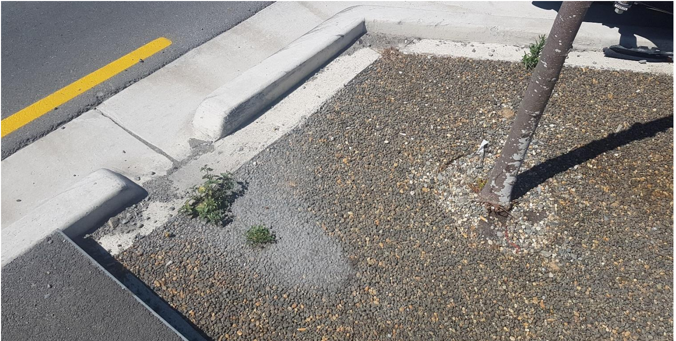
Figure 8: Clogged resin bound aggregate
