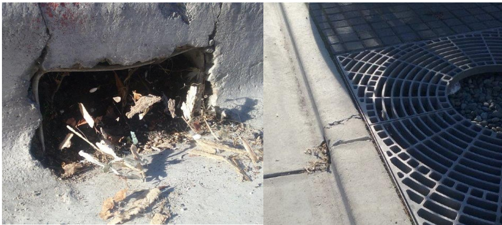
Figure 6: Kerb inlets - blocked (left) and cracked (right)
