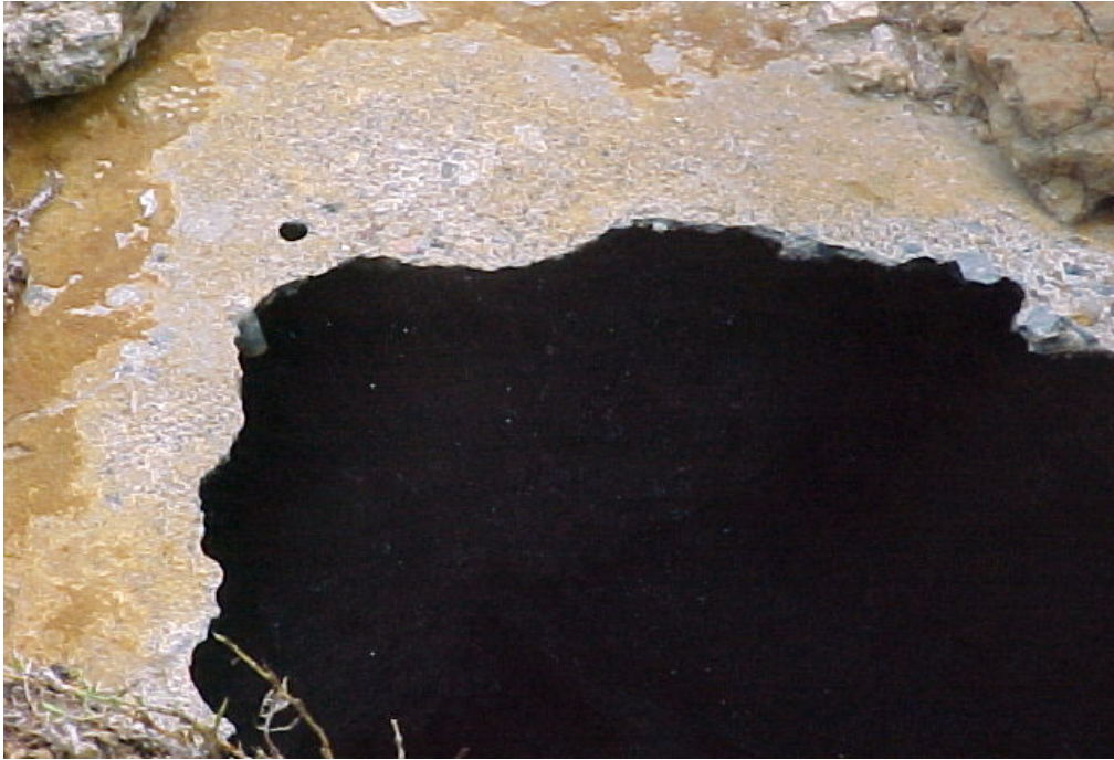
Collapsed 900 mm Gravity Main of GCW after a short service time of 12 years (Feb 2003)
