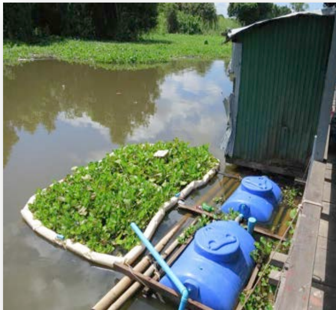
Larger HandyPod system, complete with final-stage hyacinth pond, at a floating school
