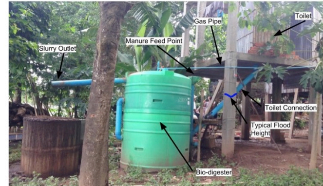
Bio-Digester installed as part of the toilet trial
