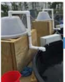
Sludge settler for biosolids (sludge) removal from BTF effluent
