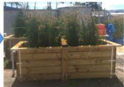
Final Surface Flow Constructed Wetland (HW) for further polishing the BTF effluent before discharge
