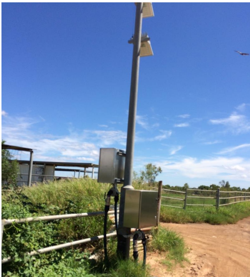
Figure 9: One of the 16 new remote irrigation actuators at Mount Isa
