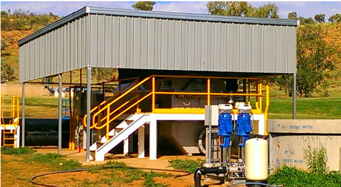
Figure 8: Mount Isa WWRP Upgrade – New Tertiary Filter
