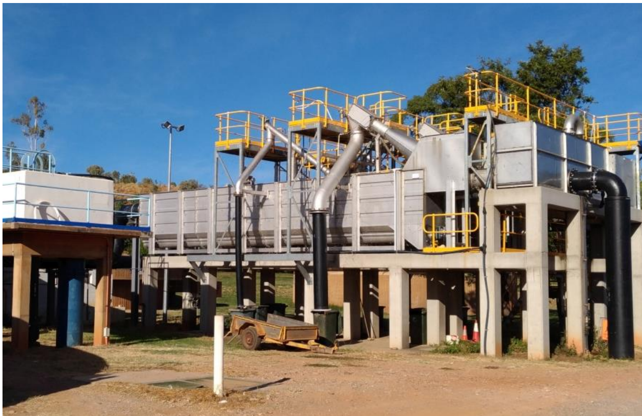
Figure 5: Mount Isa WWRP – New Inlet Works with the disused old concrete inlet channel on the left
