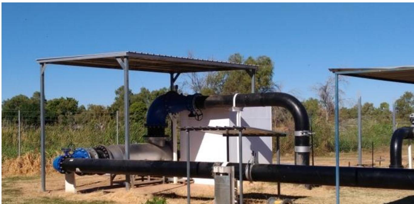
Figure 9: Mount Isa WWRP Upgrade – New UV Unit
