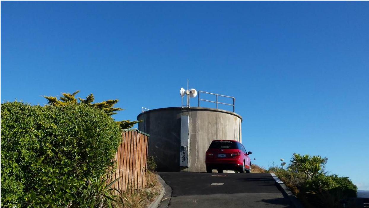
Photograph 2: a sample repeater site
