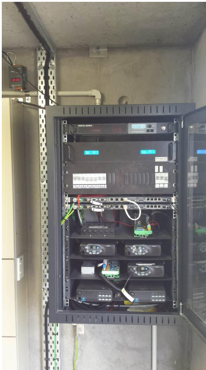
Photograph 3: A Typical Install
